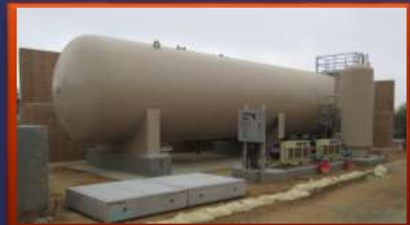
Perris PS Surge Protection
