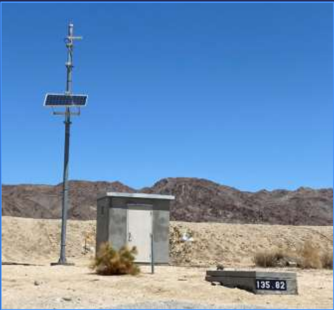
Existing Monitoring Station
