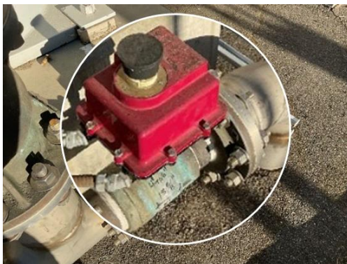
Open loop strainer valve, spool, and actuator (before replacement)
