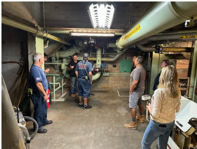
Tour with the local fire department at Gene pumping plant
