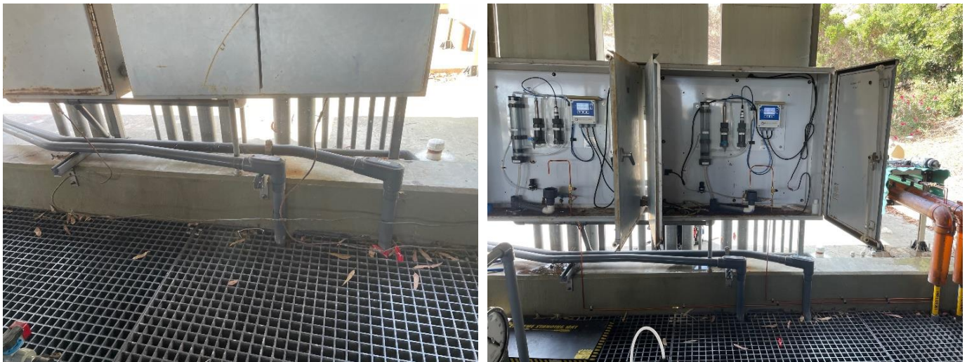
Garvey Reservoir tank farm water quality analyzers
