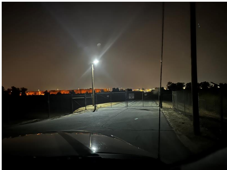
Newly installed solar light shown pre-dawn at the Chemical Unloading Facility
