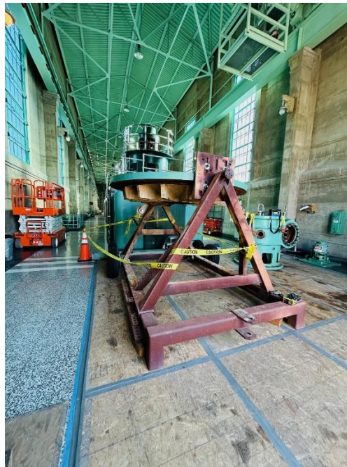
Pump cover staged on a rotisserie at the Gene pumping plant
