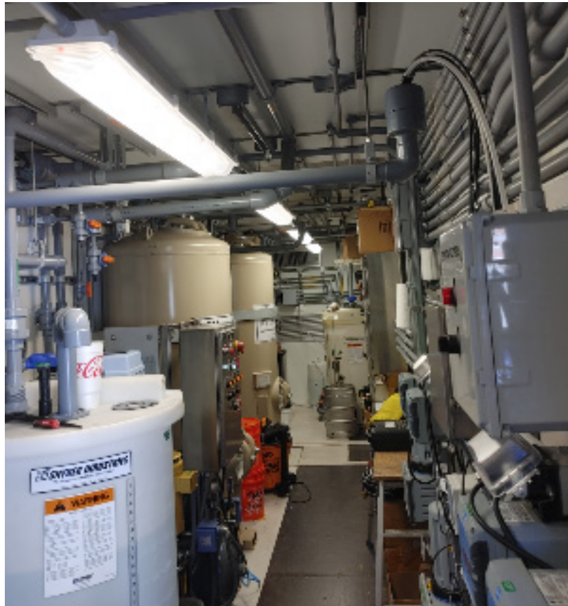
CRA Domestic Water Treatment System —Temporary Treatment Skid at Intake Pumping Plant
