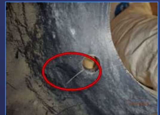
Interior Lining Crack
