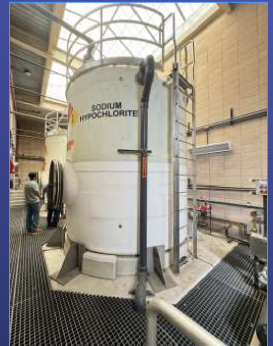
Skinner Sodium Hypochlorite Tanks
