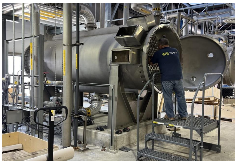
Contractor installing new dielectrics for the ozone generators at the Jensen plant
