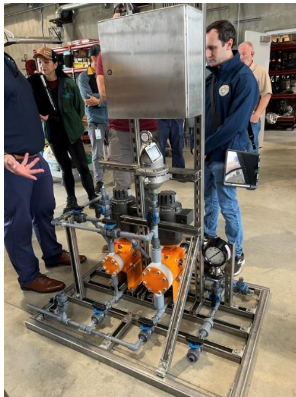
Sodium hypochlorite injection skid prototype to manage nitrification in the distribution system
