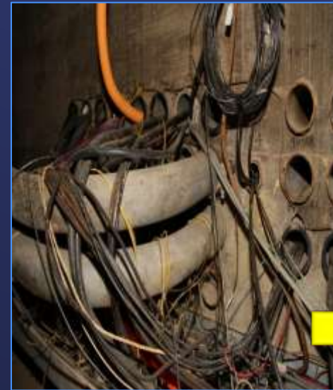
Existing Cables in Vaults
