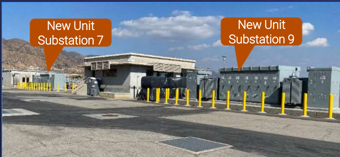
New Unit Substation
