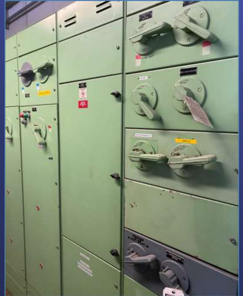
Original Plant Equipment from 1972
