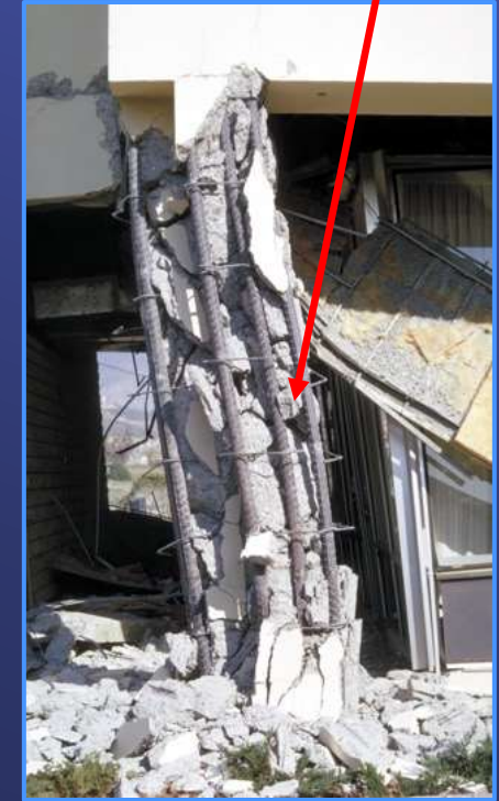
Example of Column Failure
