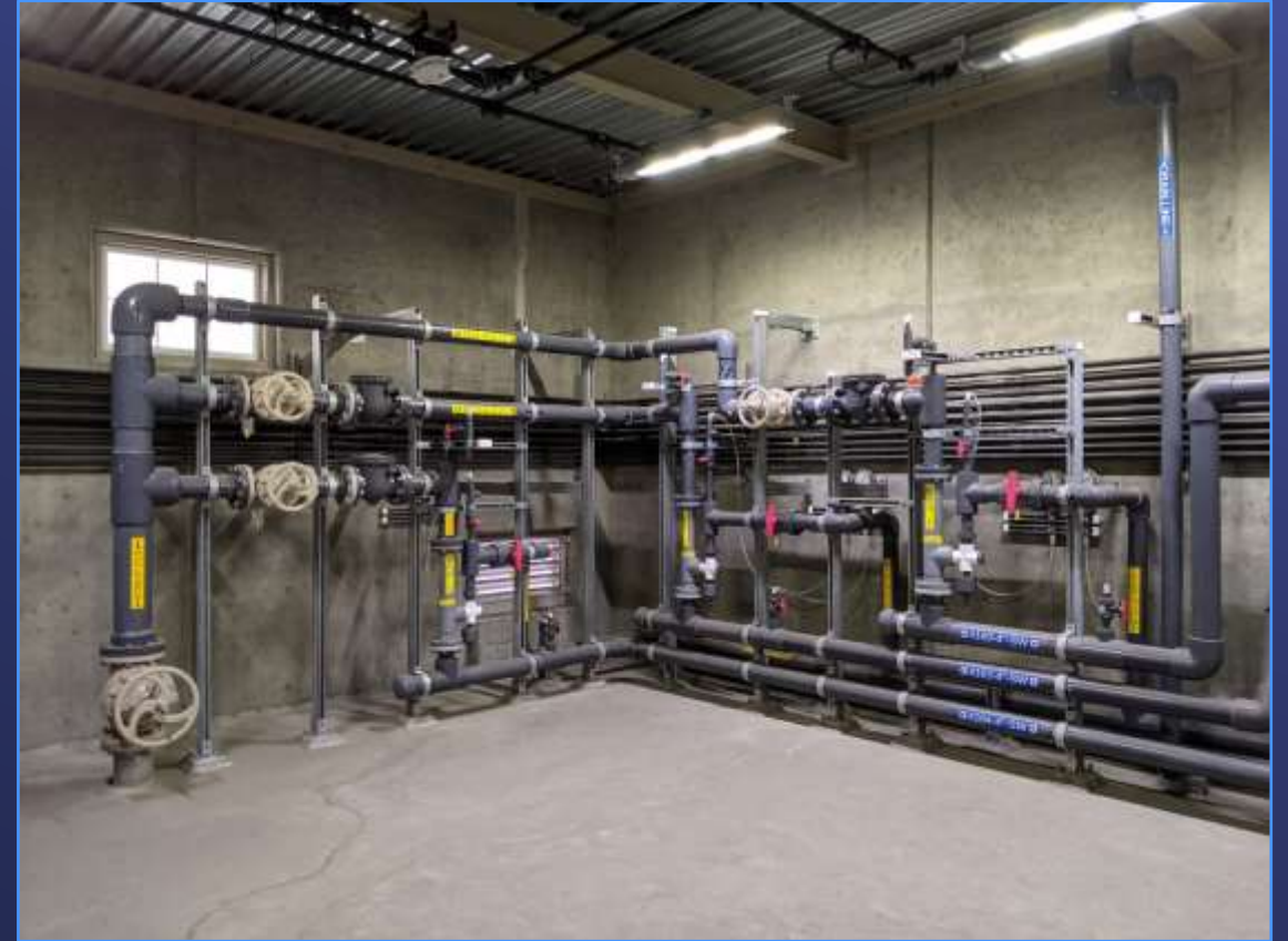
Bromate control ejector building at Weymouth
