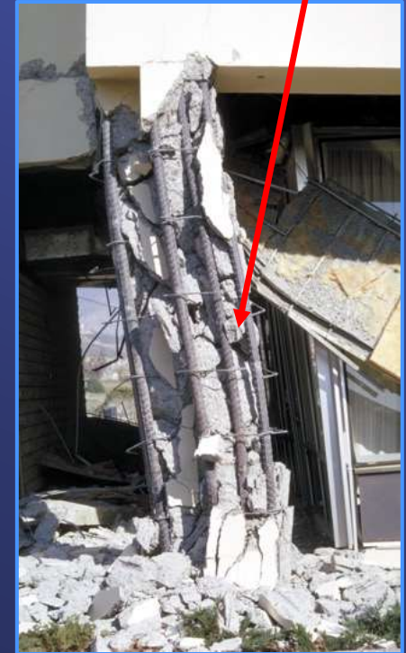
Example of Column Failure
