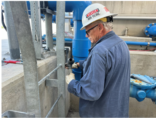
Staff installing new conduit for electrical receptacles at the Napolitano Innovation Center
