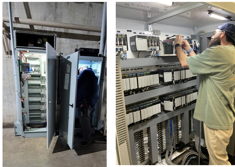
Legacy RTU controls cabinet (left) and staff working on new PLC control center (right) for Weymouth Basins 5-8
