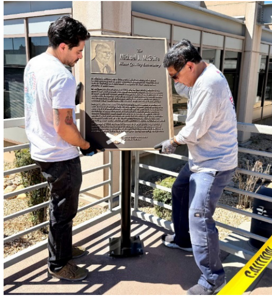
Installation of plaque commemorating the naming of the Michael J. McGuire Water Quality Laboratory
