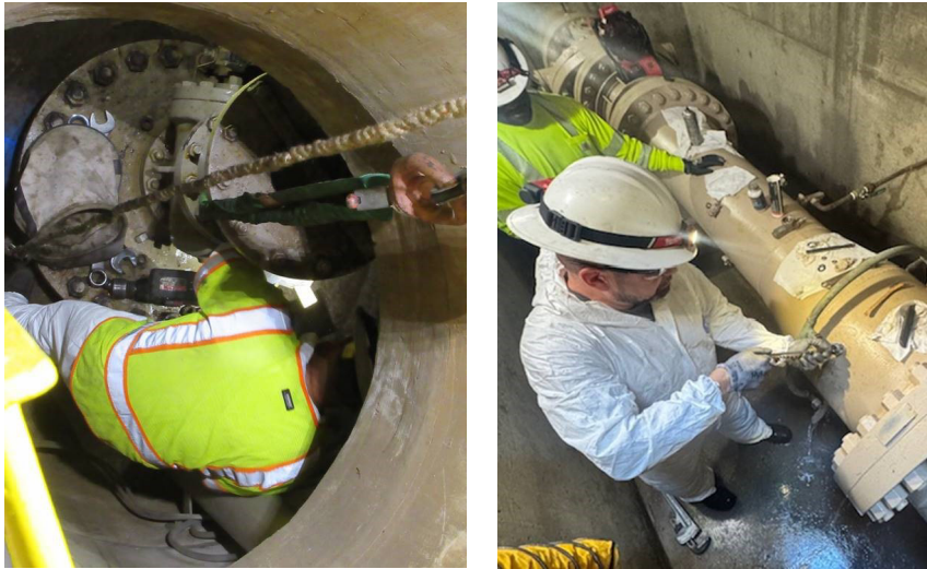
Staff removing a faulty valve (left) and performing maintenance on a service connection meter on the South Coast Feeder (right)
