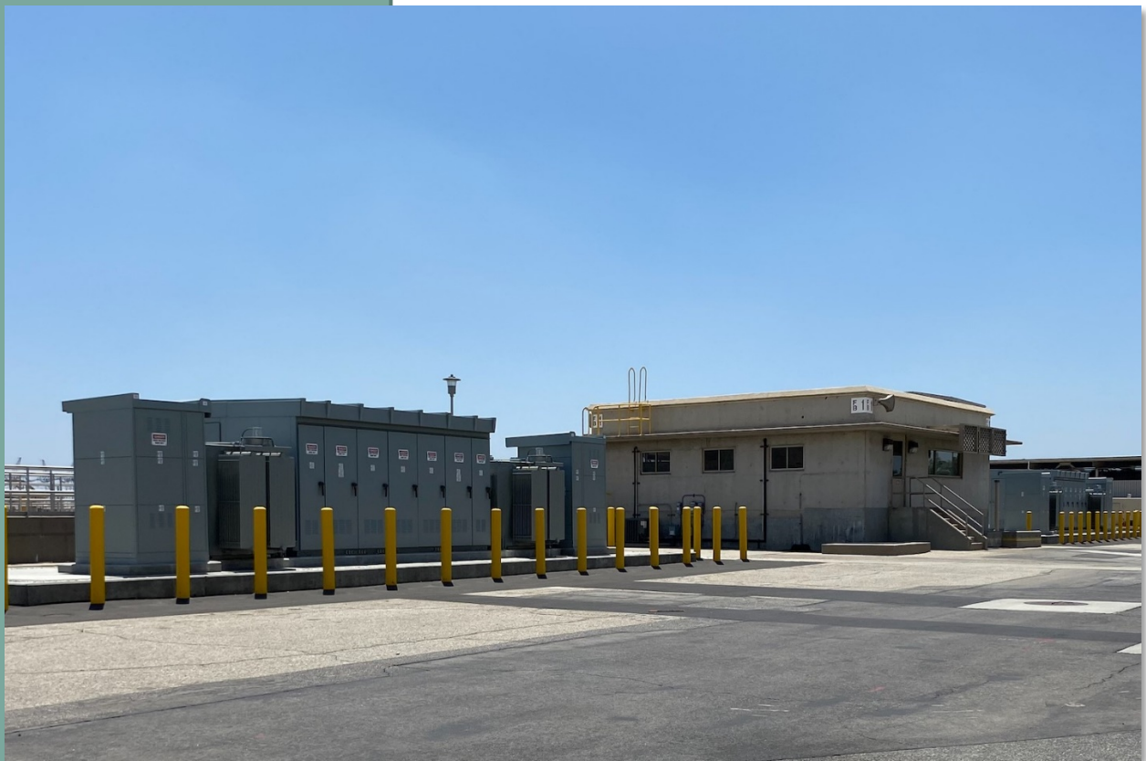
Completed unit substations 7A&B and 9A&B at the Jensen plant
