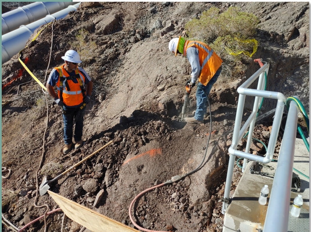
Contractor chip excavated subgrade for above ground conduit support pedestals at Intake Pumping Plant
