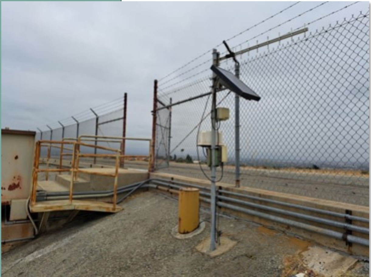
Existing dam monitoring station at Garvey Reservoir
