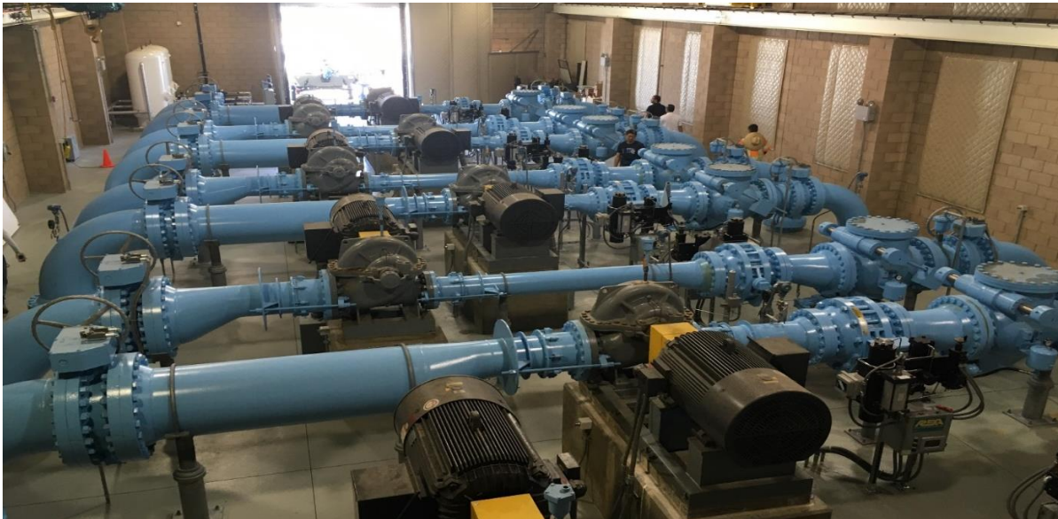
Interior of the existing SBVMWD Foothill Pump Station in the City of Highland
