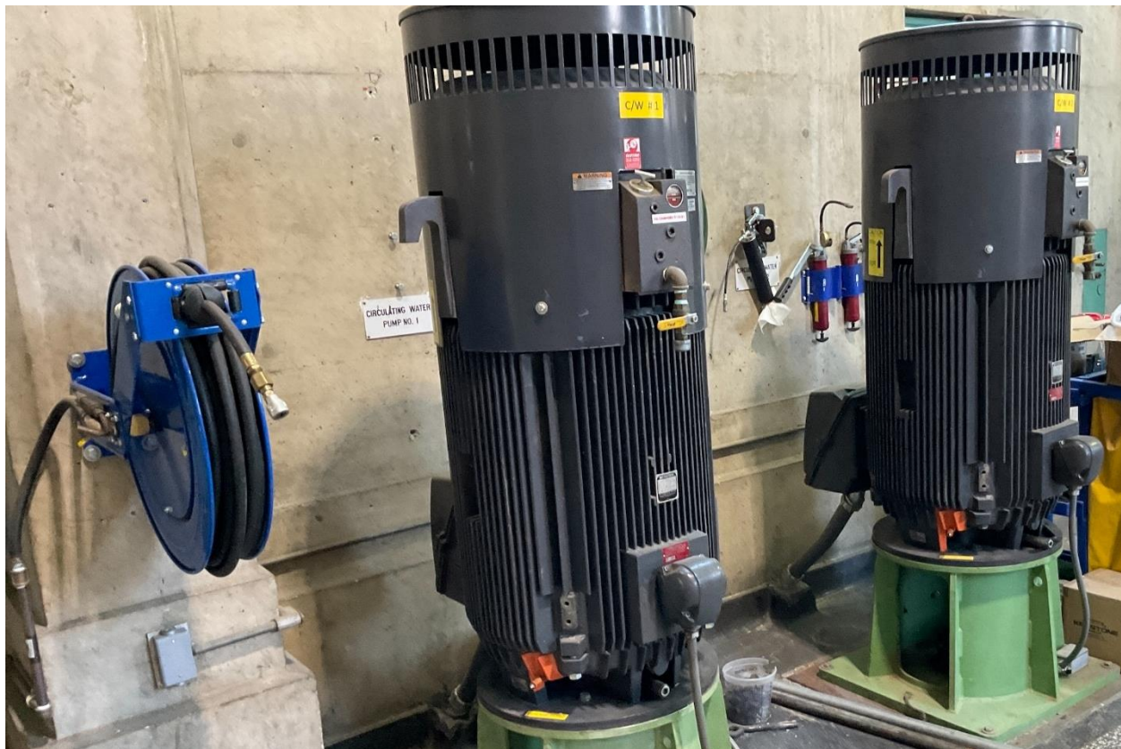
Circulating water and sump pumps at Iron Mountain Pumping Plant
