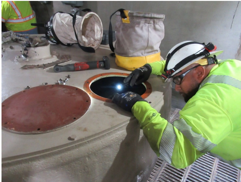
Staff inspecting the operation of a 42-inch valve during routine preventive maintenance at the Sepulveda Feeder
