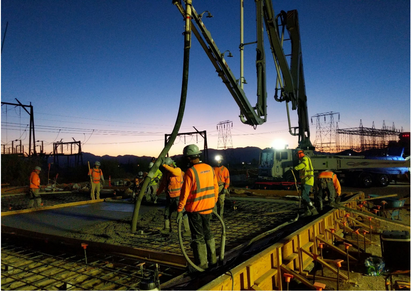
CRA Storage Buildings—Placing Concrete for Storage Building Slab at Eagle Mountain Pump Plant
