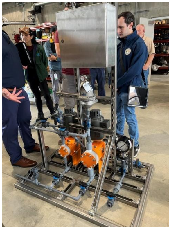
Sodium hypochlorite injection skid prototype to manage nitrification in the distribution system
