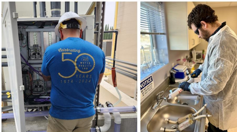
Electrical panel maintenance (left) and preparing ultrafilters for microbial sampling of the MBRs (right) at the NIC demonstration facility
