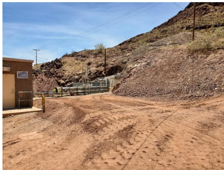
New crane pad for better access to perform maintenance
