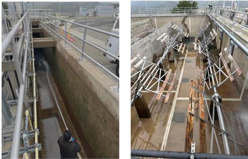
Staff washing down the sedimentation basin and influent channel at the Diemer plant
