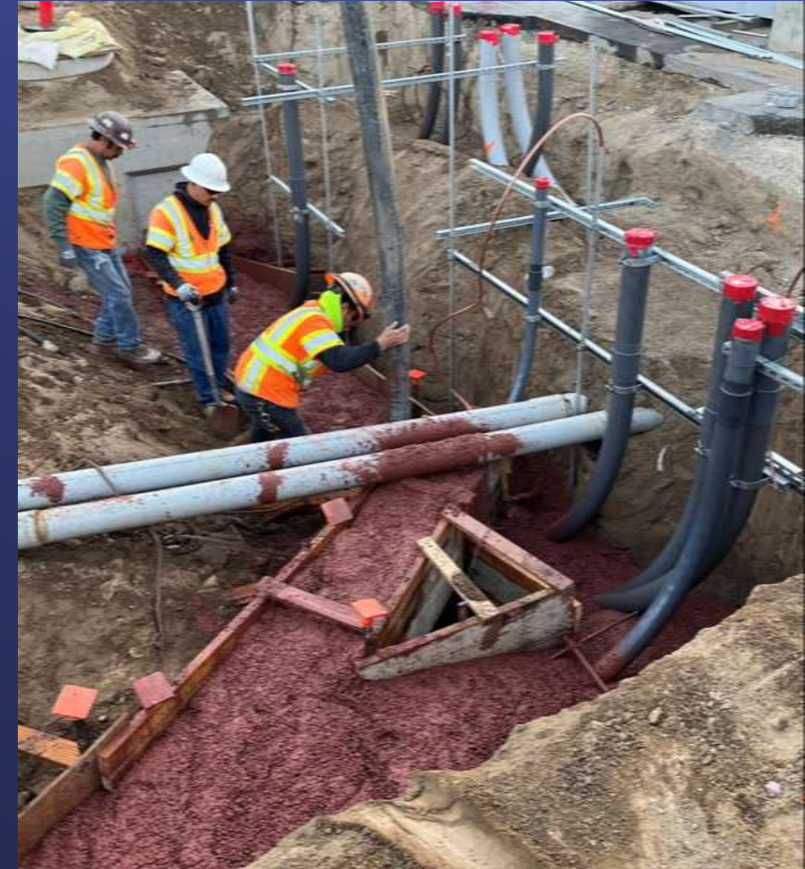
Electrical Duct Bank
