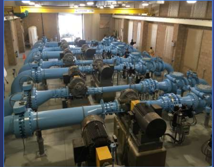
Existing Foothill Pump Station
