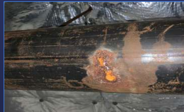
Externally- presenting corrosion buildup on existing fire sprinkler piping
