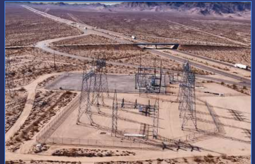
Camino Electrical Switching Station
