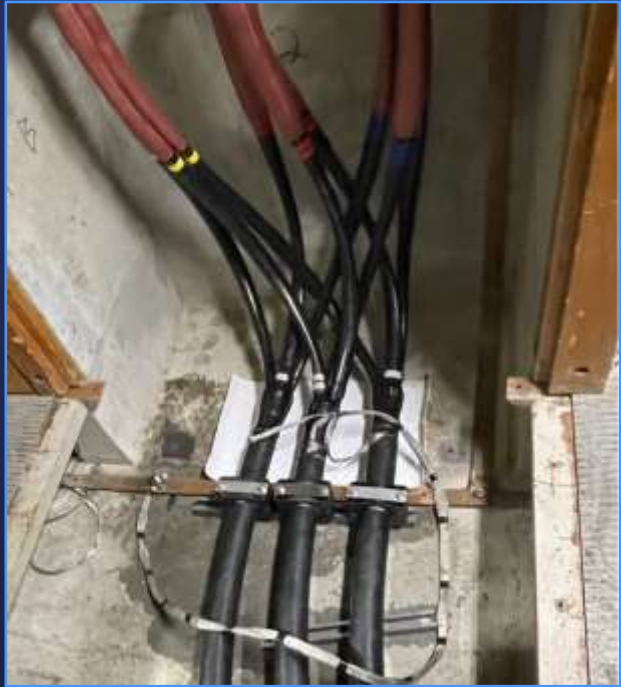
W.A. Chester LLC Terminated Cable
