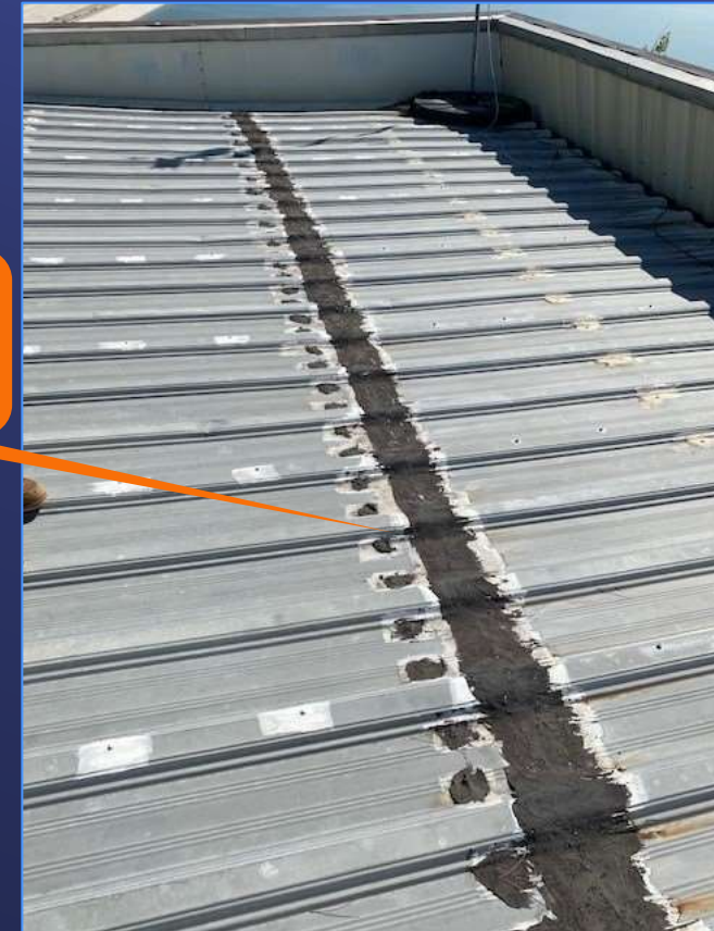
Deteriorating Metal Roof & Temporary Roof Repairs
