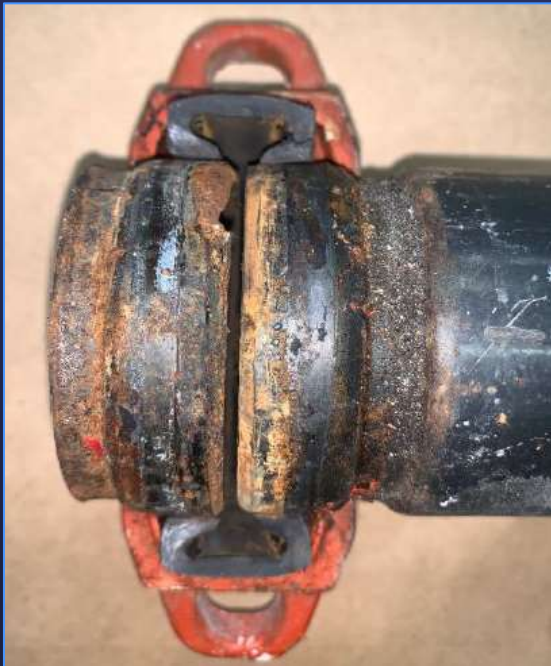
Pipe End Condition
