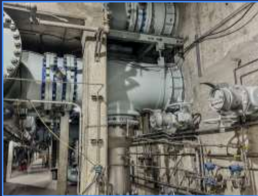
Rehabilitated Filter Valve
