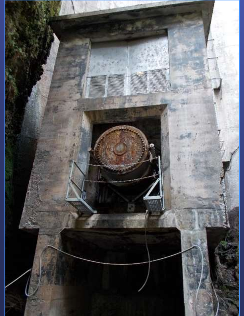
Existing Copper Basin Discharge Valve Structure
