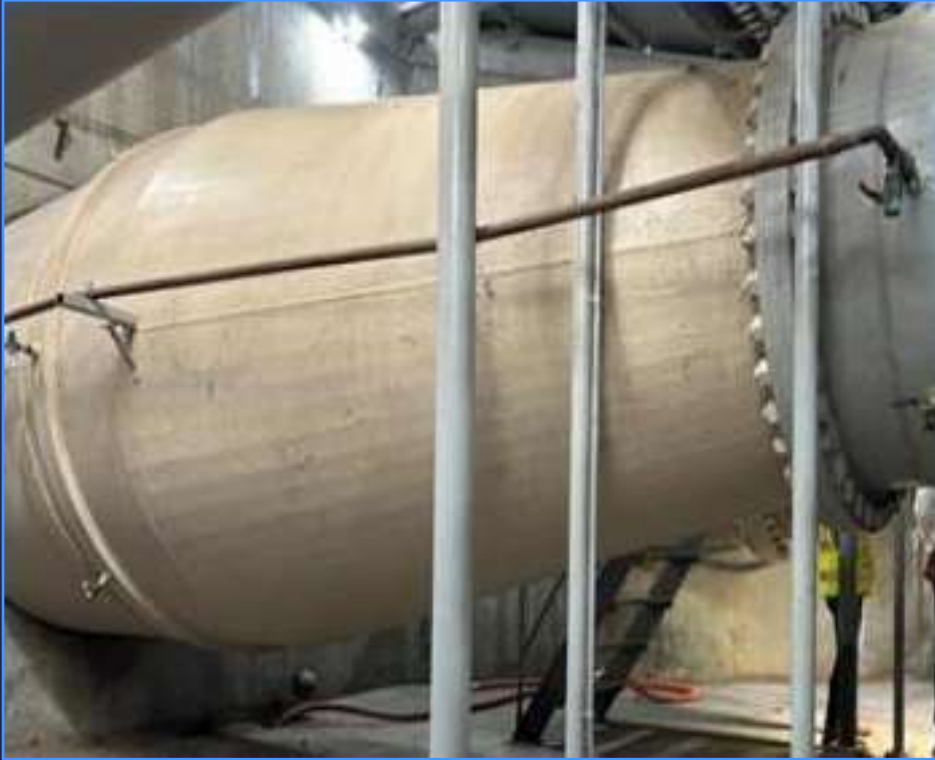
Existing 84-inch LA-17C Venturi Flowmeter in the City of Los Angeles
