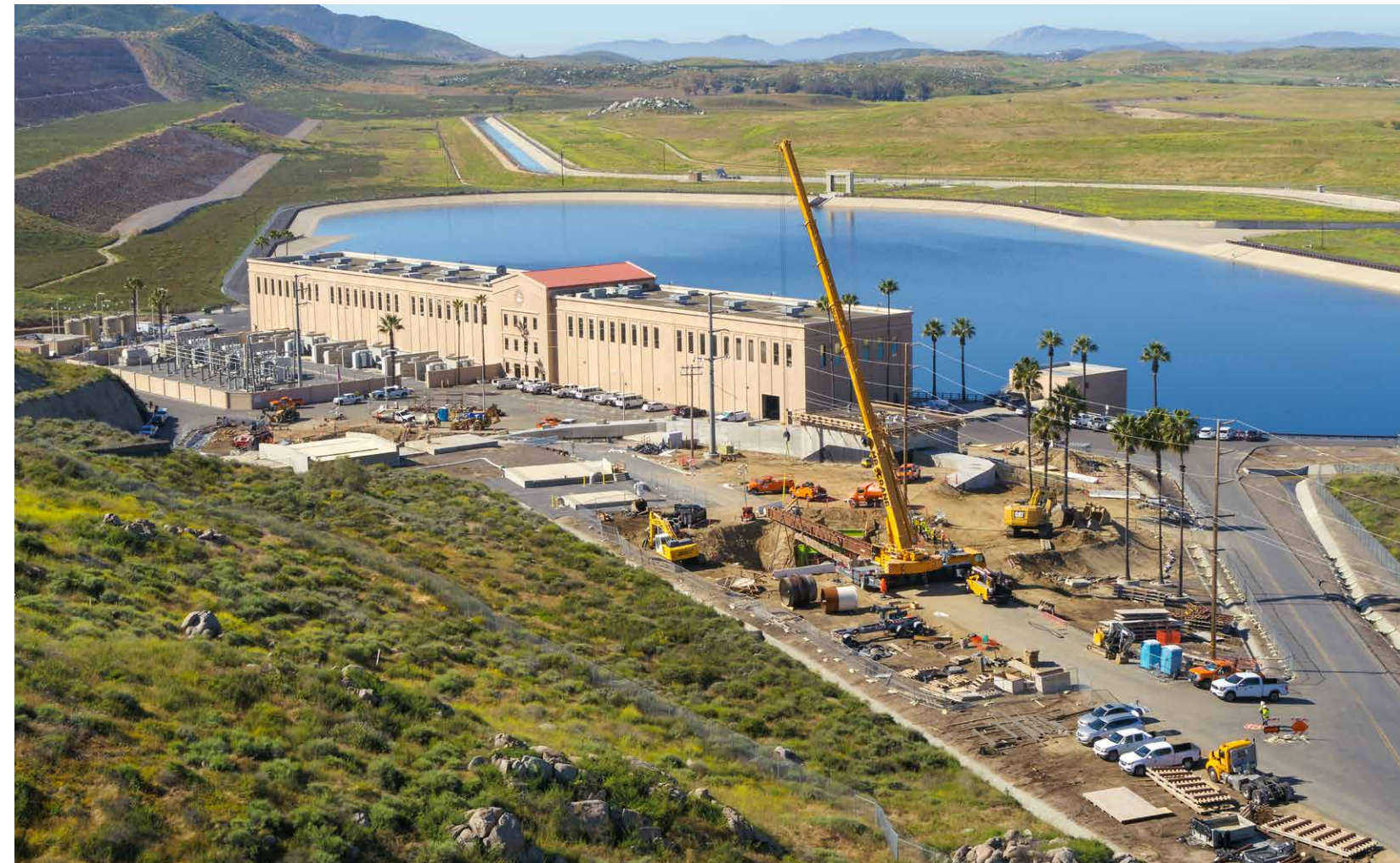
The Wadsworth Pumping Plant Eastside Pipeline Intertie project brings greater flexibility to Metropolitan's delivery system.
