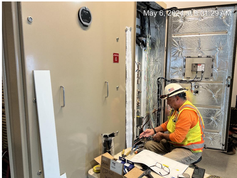
Termination of Power Supply Control Wires
