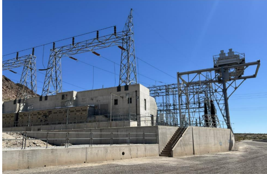
Hinds Pumping Plant Switch House
