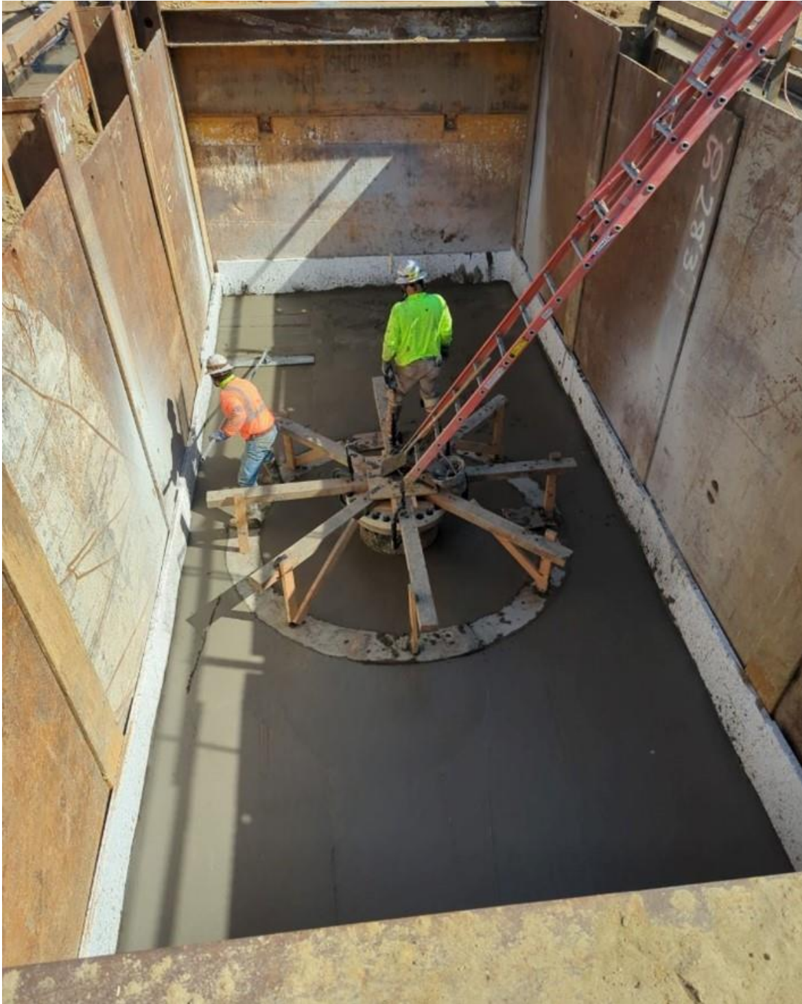
Placement of concrete encasement for the pipe closure piece in the City of Irvine performed under Stage 1
