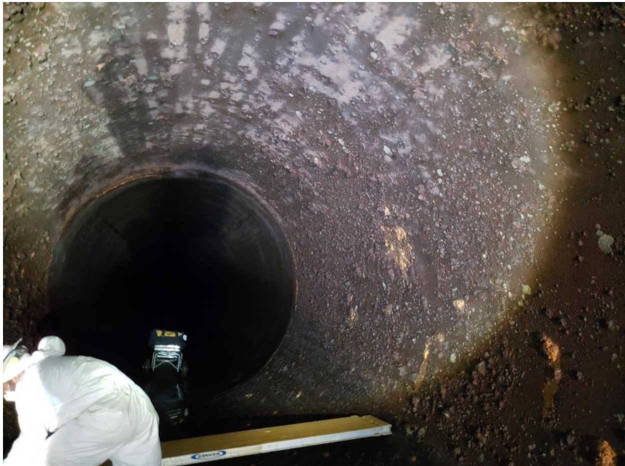
Performing inspection of 120-inch diameter steel pipe with missing mortar lining
