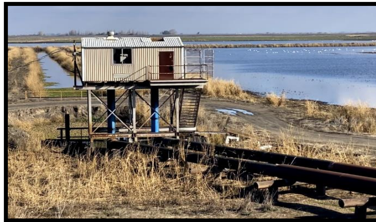
Figure 11 – Delta Island Pump Discharge Station 53
