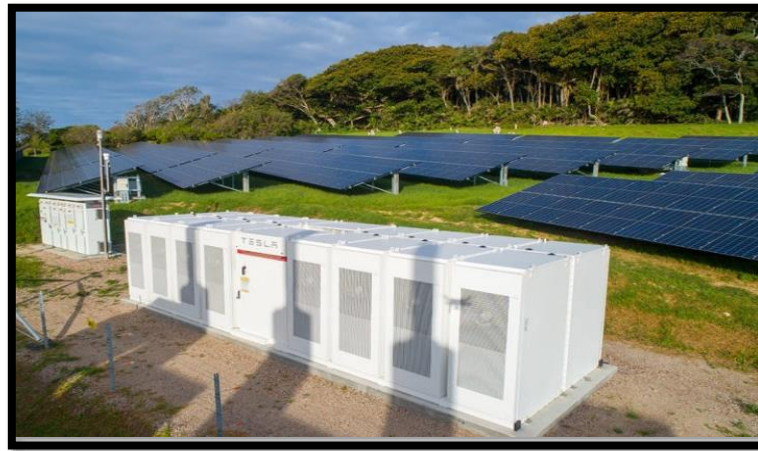
Figure 10 – Small Scale Solar Microgrid with Battery Energy Storage System 51
