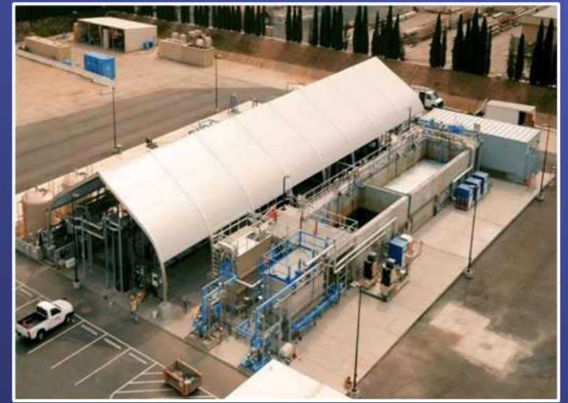
Pure Water Southern California Demonstration Plant
