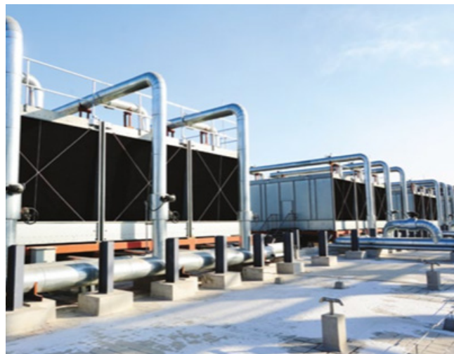
Cooling Tower Efficiency Improvement Funded by WSIP
