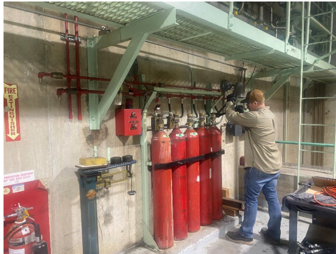
Staff replacing hoses on the Hinds pumping plant carbon dioxide fire suppression system
