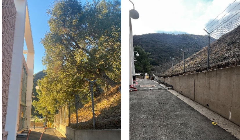
Before (left) and after (right) photos of tree and shrub removal at Sepulveda PCS
