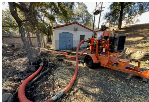
Staff provided a six-inch pump and assisted with initial startup for Pasadena Water & Power
