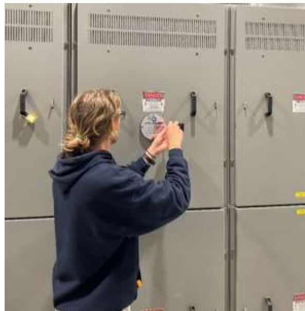
Staff installing infrared scanning windows onto high-voltage equipment at the Skinner plant
