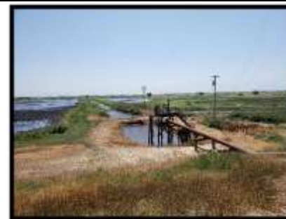
Pumping facility at Webb Tract
