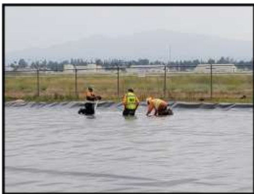
Construction contractor placing a liner for soil storage for Perris Valley Pipeline Project
