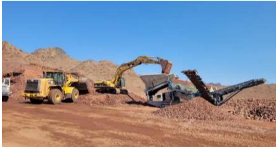
Staff processing base material through a screening machine for separation into various size aggregate at a Desert facility
