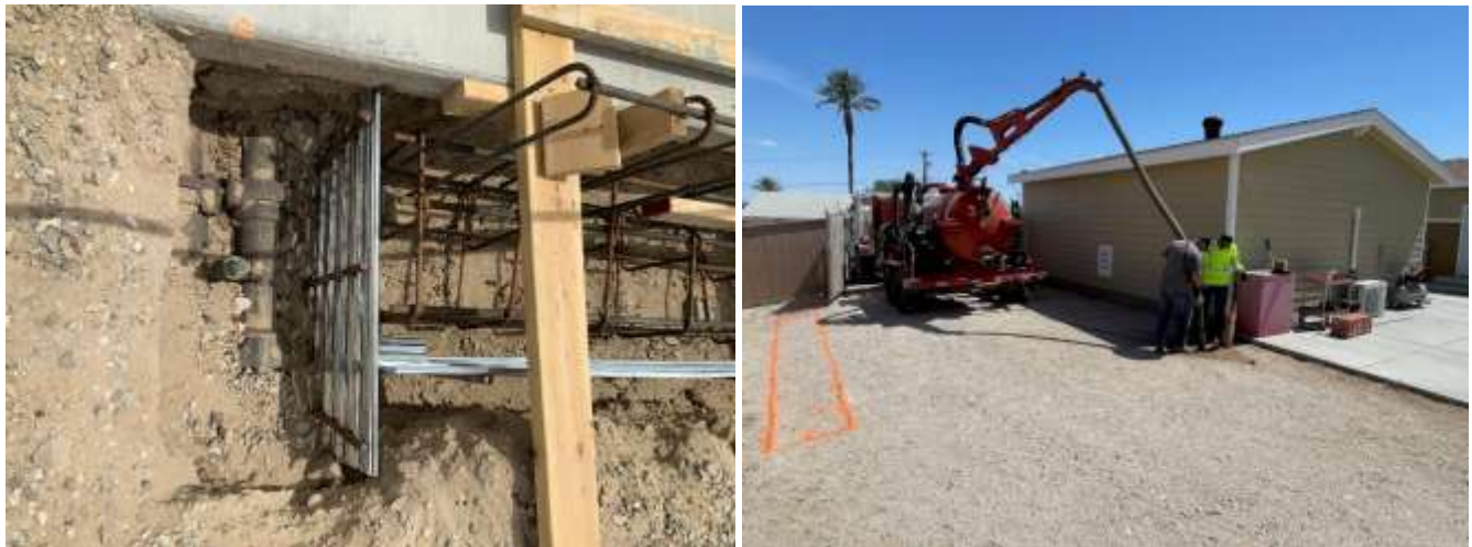
Footing formed to protect utility (left) and staff potholing buried utilities (right) at a Desert housing unit
