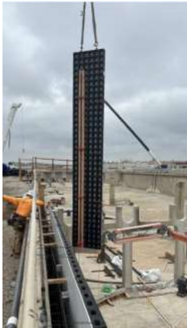
Weymouth Basins 5–8 and Filter Building No. 2 Rehabilitation Installation of Concrete Placement Panels
