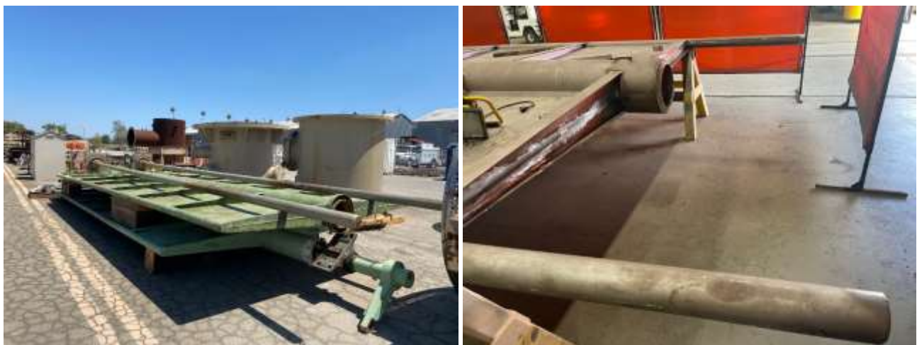
As received condition of wing gates (left) and removal of corroded gate components (right) for DWR
