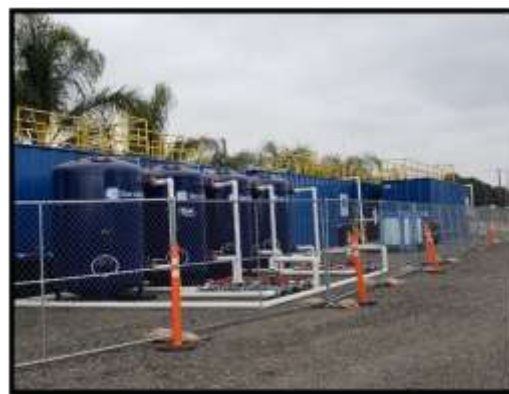
Granular activated carbon (GAC) treatment plant to filter groundwater for Perris Valley Pipeline Project
