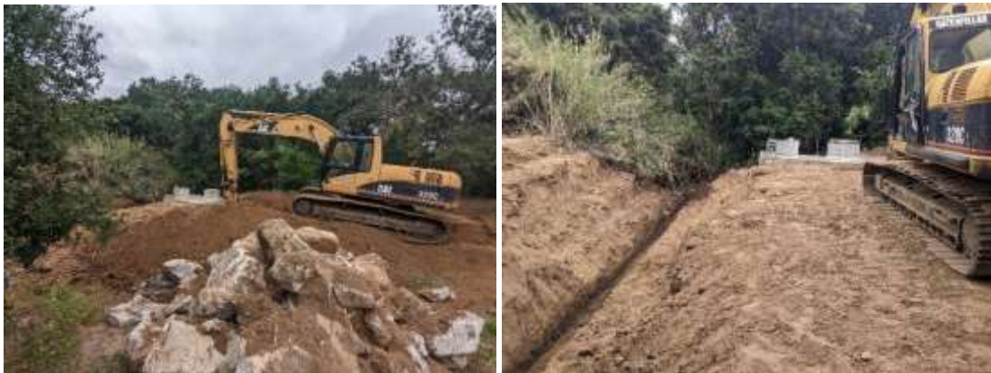
Staff using an excavator to complete the trench for the culvert along San Diego Pipelines 4 and 5
