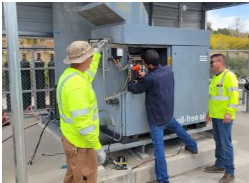
New apprentice observing electrician removing wiring (de-energized equipment) for compressor replacement at the Mills plant
