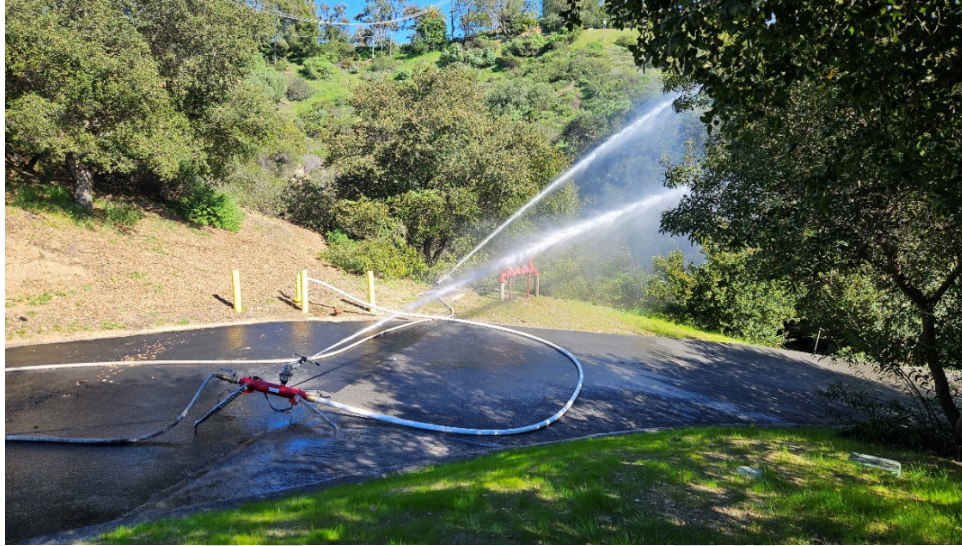
Demonstration of high-pressure water sprinklers at Eagle Rock Facility
