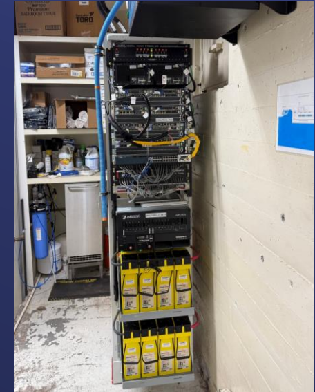
Completed Installation of MFE Microwave Radio at Intake PP
