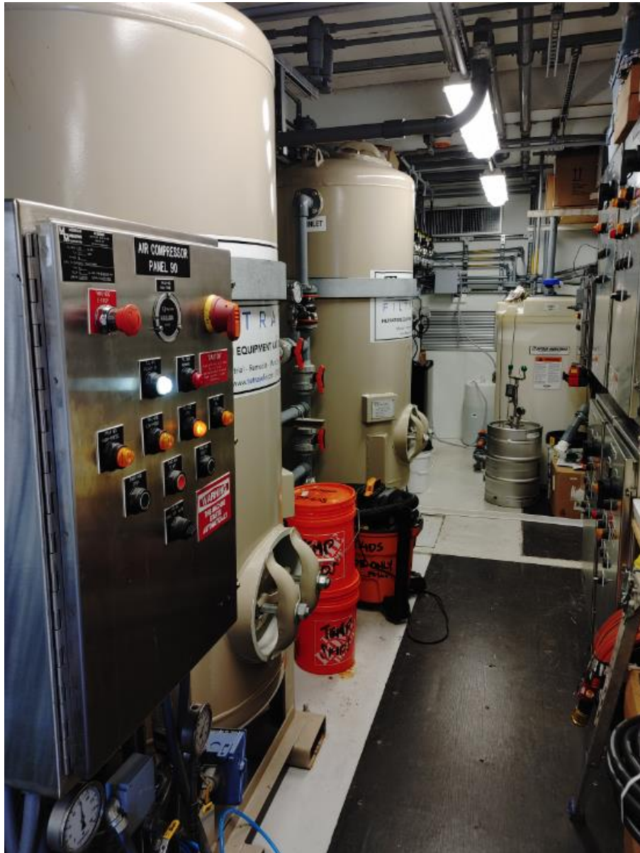
CRA Domestic Water Treatment Systems Upgrade — Temporary Treatment Skid at Intake Plant
