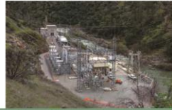
⚡ New Colgate Powerhouse
