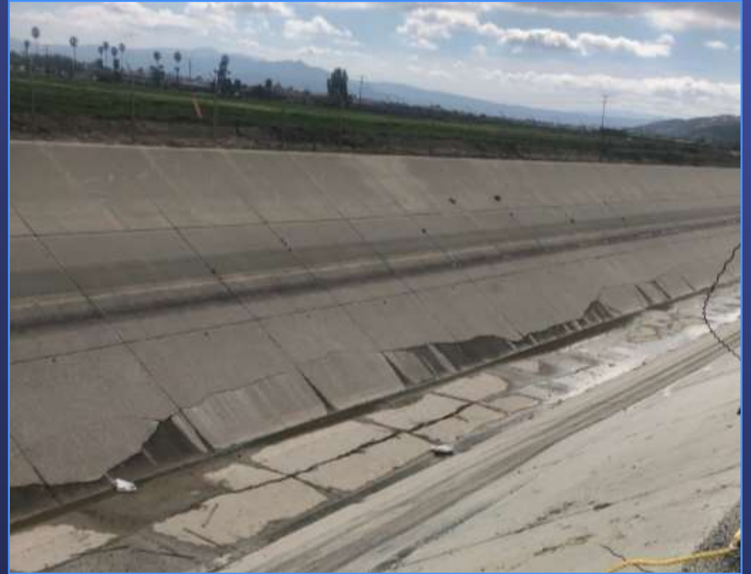
Damaged concrete liner
