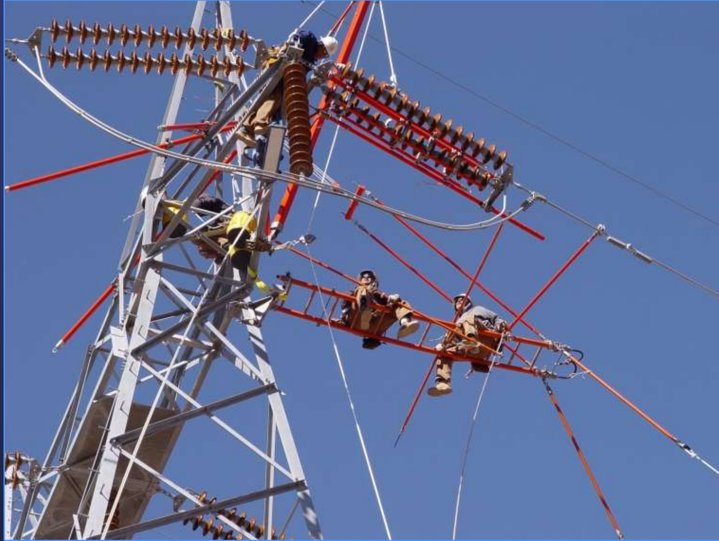
230kV Power Line
