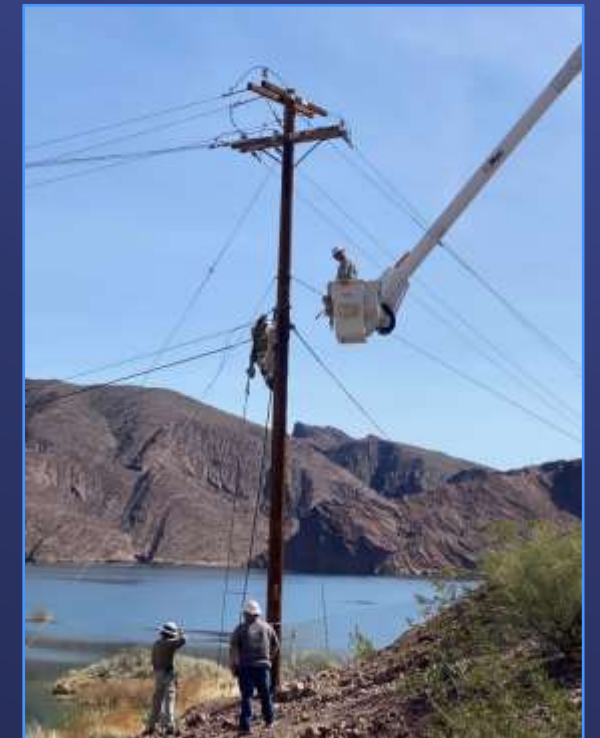
Copper Basin 2400V System Isolation
