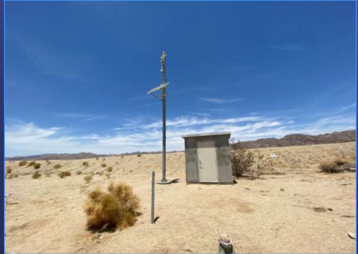
Flow Monitoring Stations (Planned completion: 2024) $5.3M
