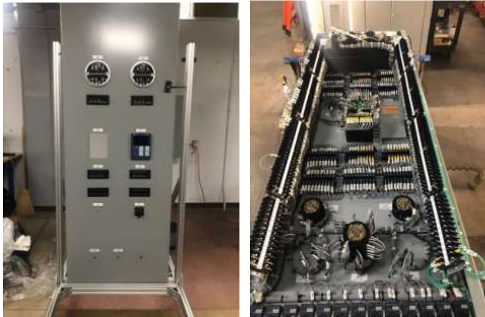
Front of transformer protection panel (left) and completed wiring in the back of the panel (right) at Hinds pumping plant
