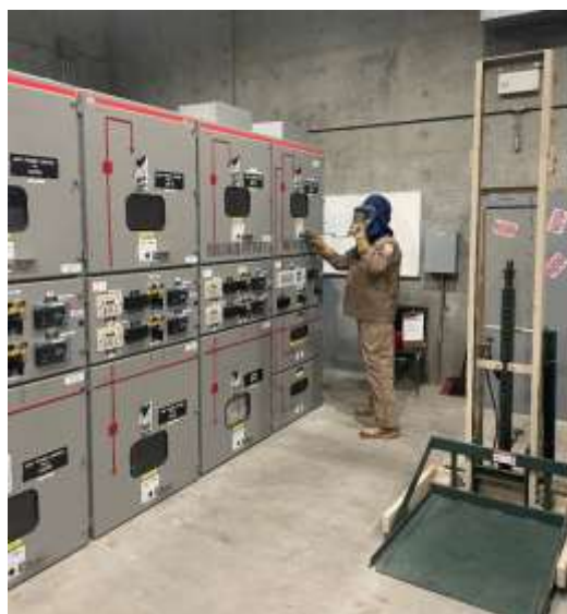
Staff performing high-voltage switching to accommodate arc flash data gathering at the Skinner plant
