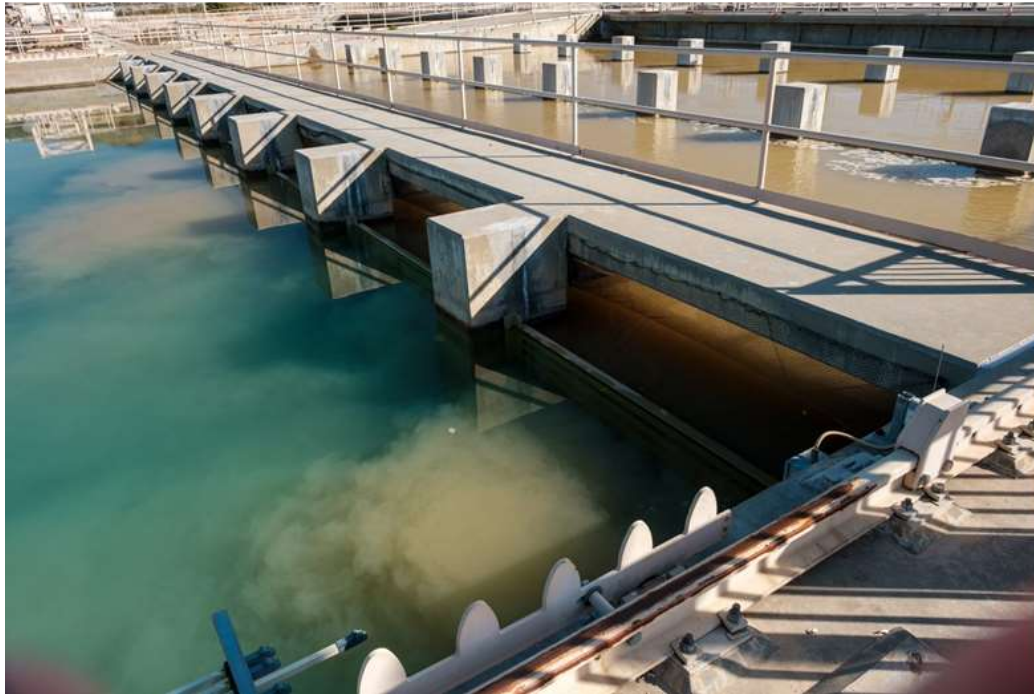
Turbidity from Castaic Lake being removed during the treatment process at the Jensen plant
