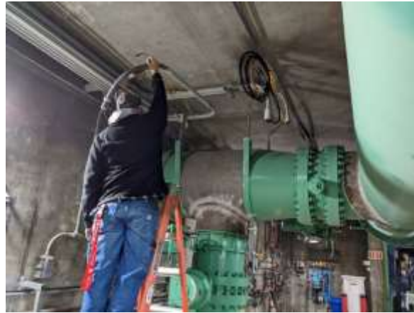
Staff preparing for repairs of the backwash header at the Diemer plant
