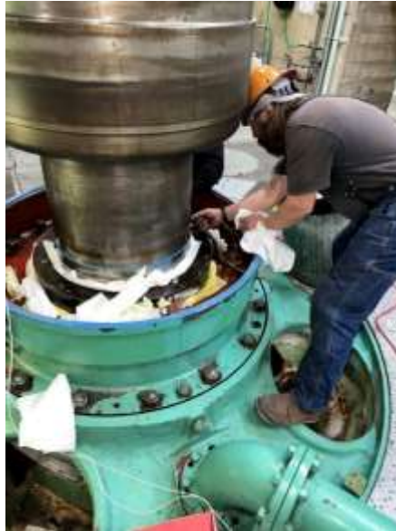
Staff replacing an RTD on a pump bearing at Eagle Mountain pumping plant
