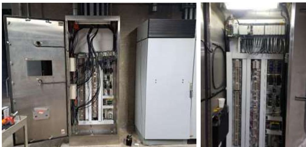
Previous PLC control panel (left) and new Allen Bradley PLC 5000 controller (right) at the Mills plant
