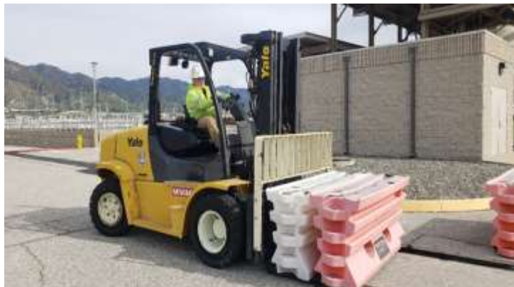
Staff installing traffic control barriers to protect the temporary solids handling pipeline
