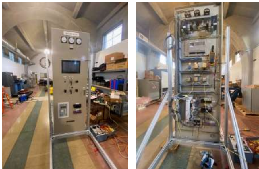
Front of AVR Panel (left) and completed wiring in the back of the panel (right) at Red Mountain HEP
