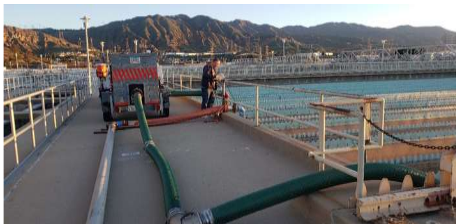
Staff reviewing installation of a temporary solids handling pipeline at the Jensen plant
