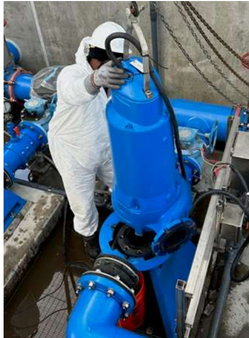
Staff installing a replacement return activated sludge pump at the PWSC demonstration plant
