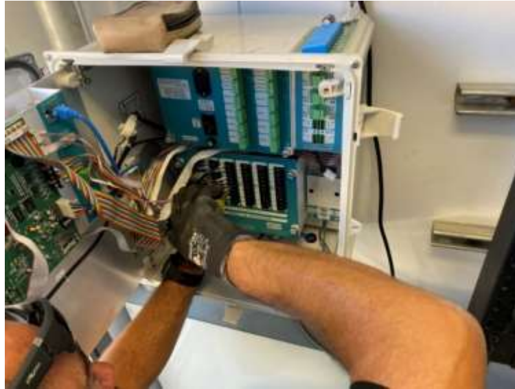
Staff troubleshooting a flowmeter at Hinds pumping plant
