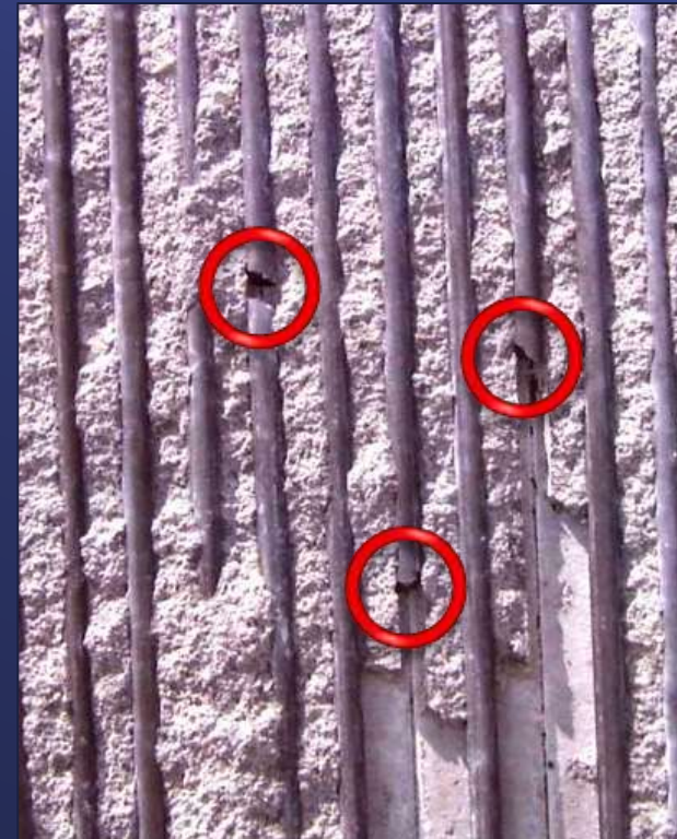
Broken Prestressing Wires
