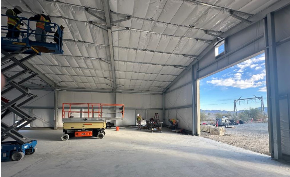
CRA Storage Buildings—Contractor staff installing overhead conduit at the interior of the Storage Building at Eagle Mountain Pumping Plant
