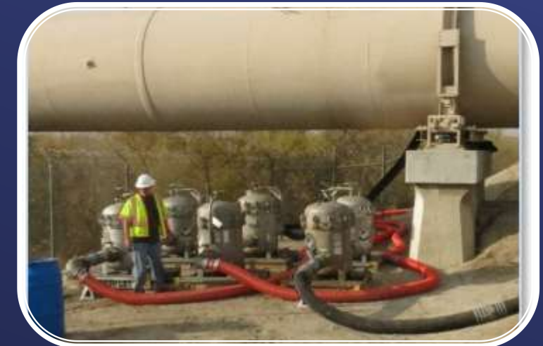
Control Measures (e.g., Filtration) during Raw Water Discharges
