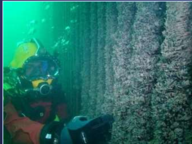
Colonized Intake Trash Rack
