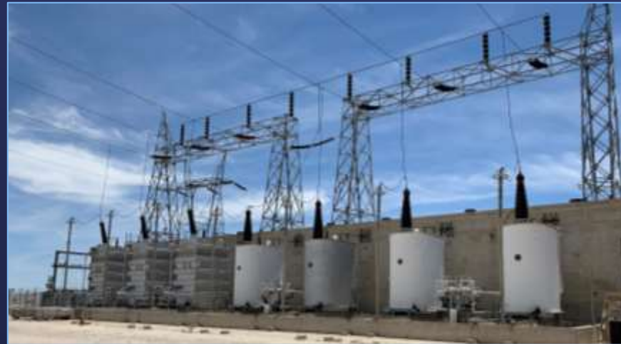
Iron Mtn. Pumping Plant
