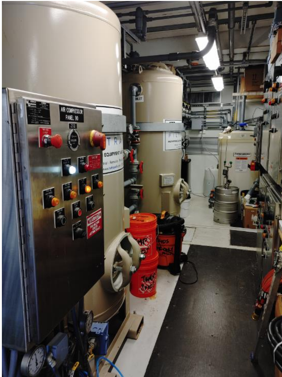
CRA Domestic Water Treatment Systems Upgrade — Temporary Treatment Skid at Intake Plant
