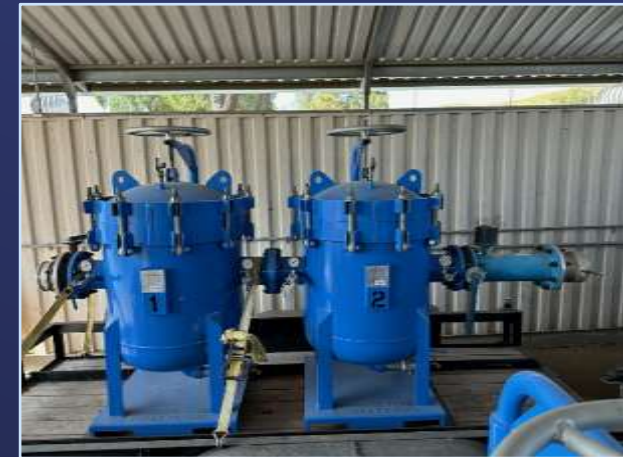
Filters for Raw Water Discharges
