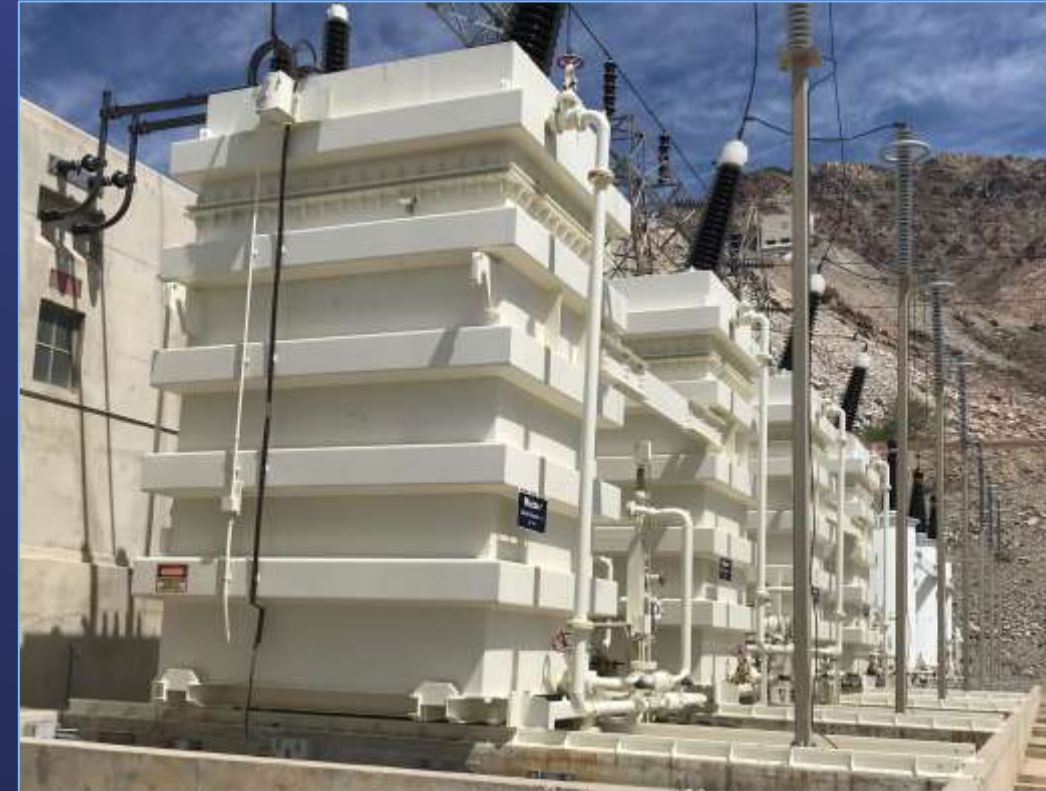
Eagle Mtn. Pumping Plant
