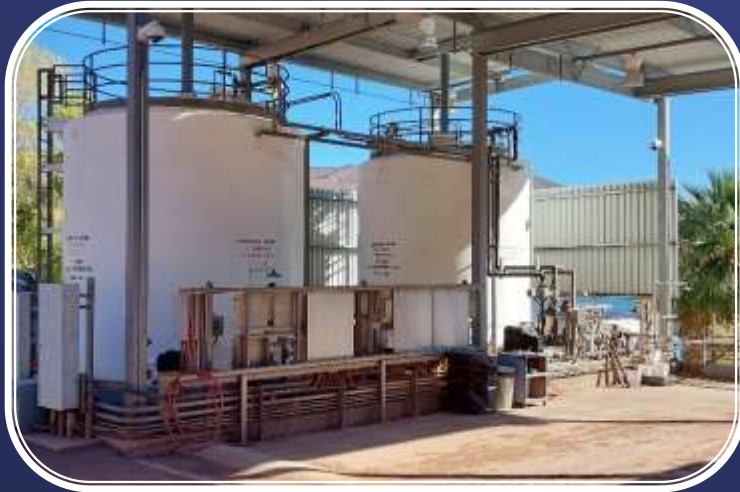
Continuous Chlorination at Copper Basin, Lake Mathews, Lake Skinner
