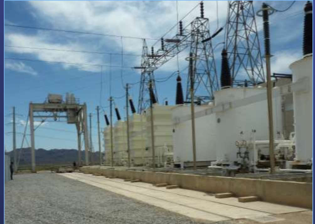
Hinds Pumping Plant
