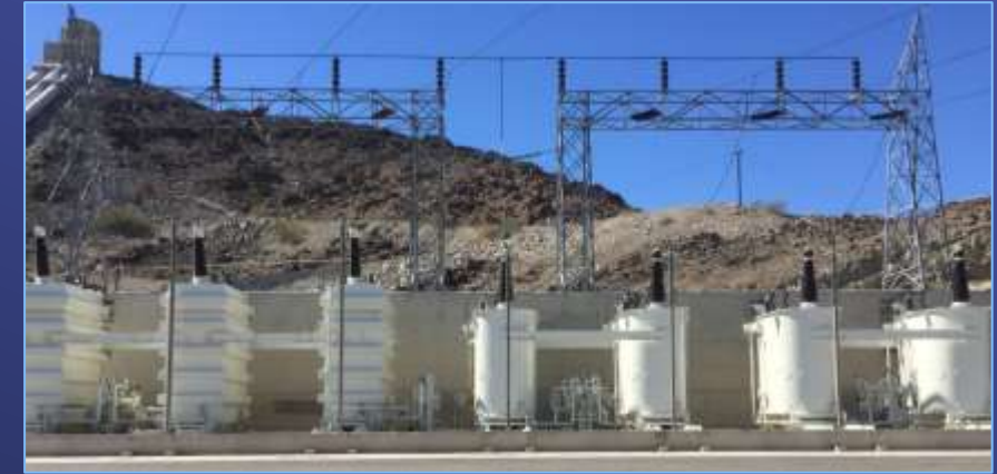
Eagle Mtn. Pumping Plant
