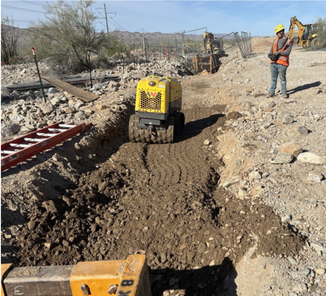
CRA Eagle and Hinds Utilities Hinds Crew using a Walk-behind Roller Compactor to Consolidate Material
