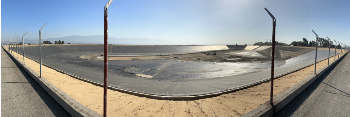
Garvey Reservoir Rehabilitation Completed Demo and Peel Back on Reservoir Floor, Facing North
