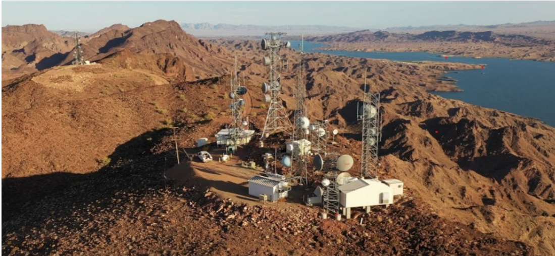
Black Metal Mountain Communications Site
