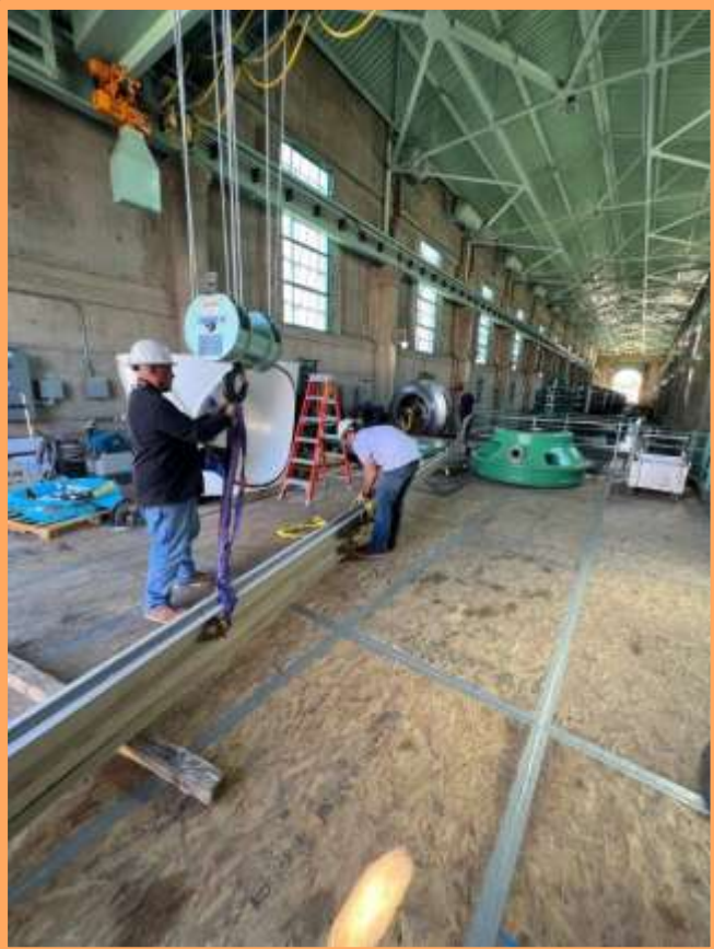
Iron Mountain – Crew using new crane during CRA pump and discharge valve rehab work
