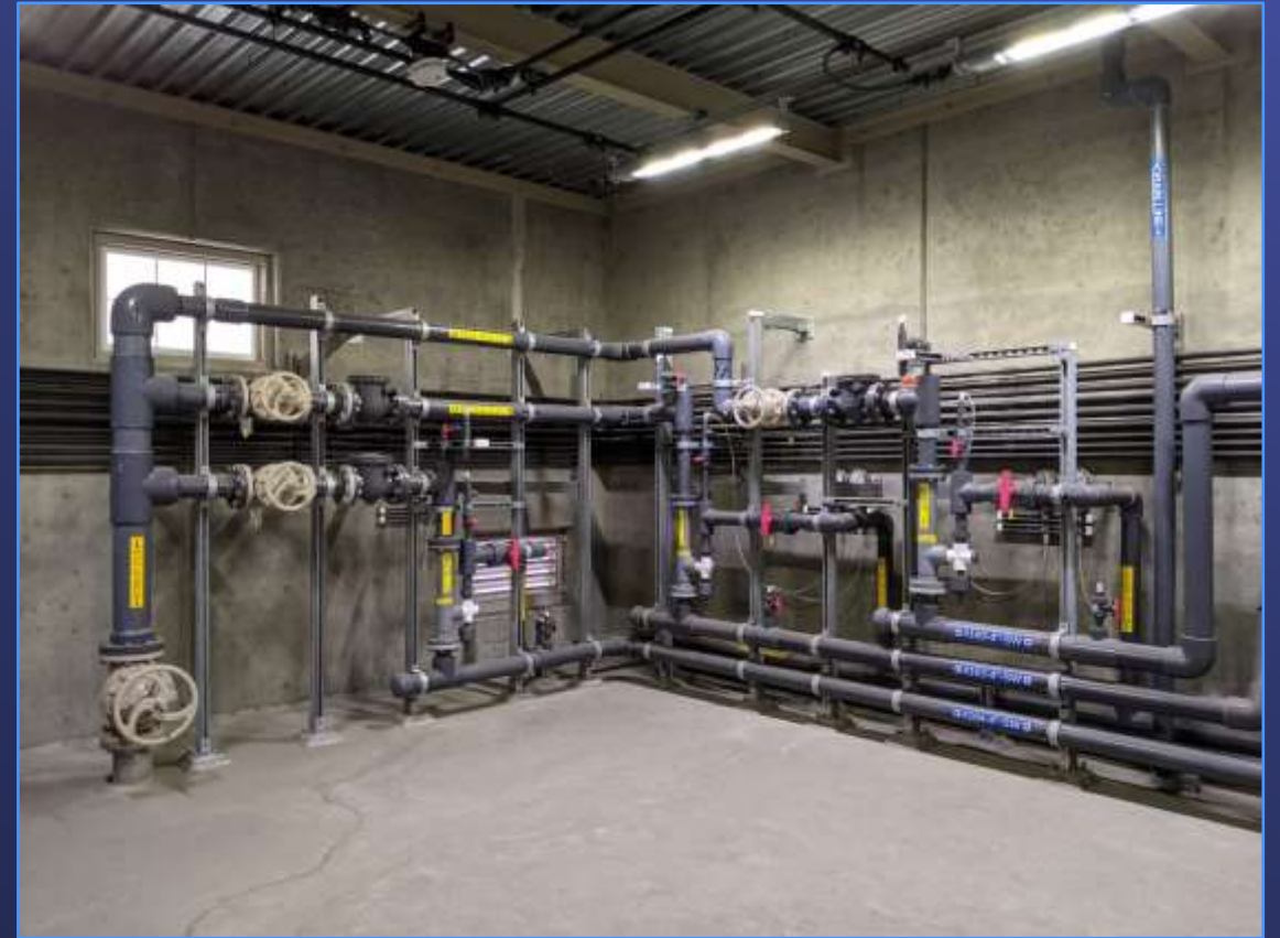
Bromate control ejector building at Weymouth
