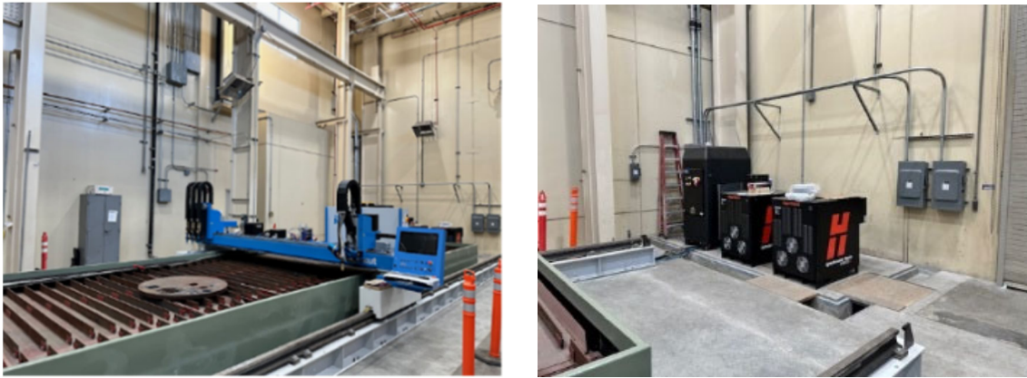
Partially installed Plasma Arc Cutting System at the La Verne Fabrication Shop
