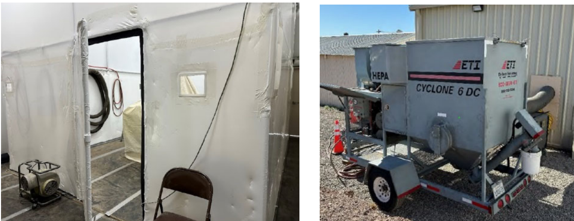
Abrasive blasting booth and dust collector to be used at Desert facilities
