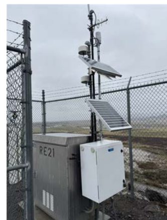
New monitoring equipment at Diamond Valley Lake
