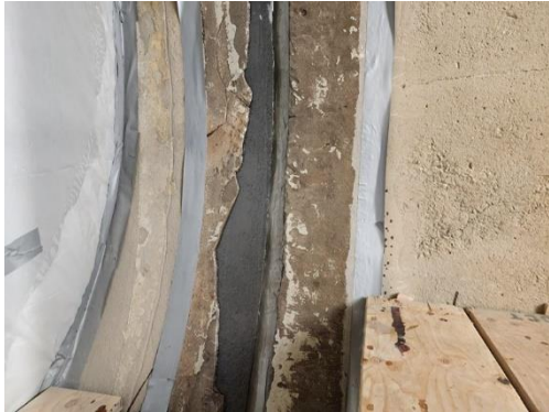
Eagle Delivery Line 2 steel to concrete transition caulking joint deterioration
