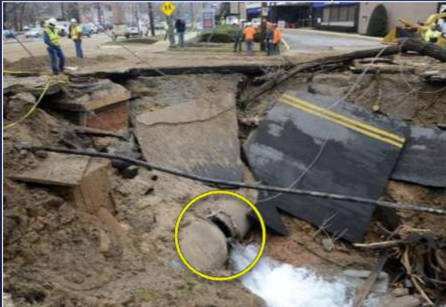
Maryland PCCP Rupture (2013)
