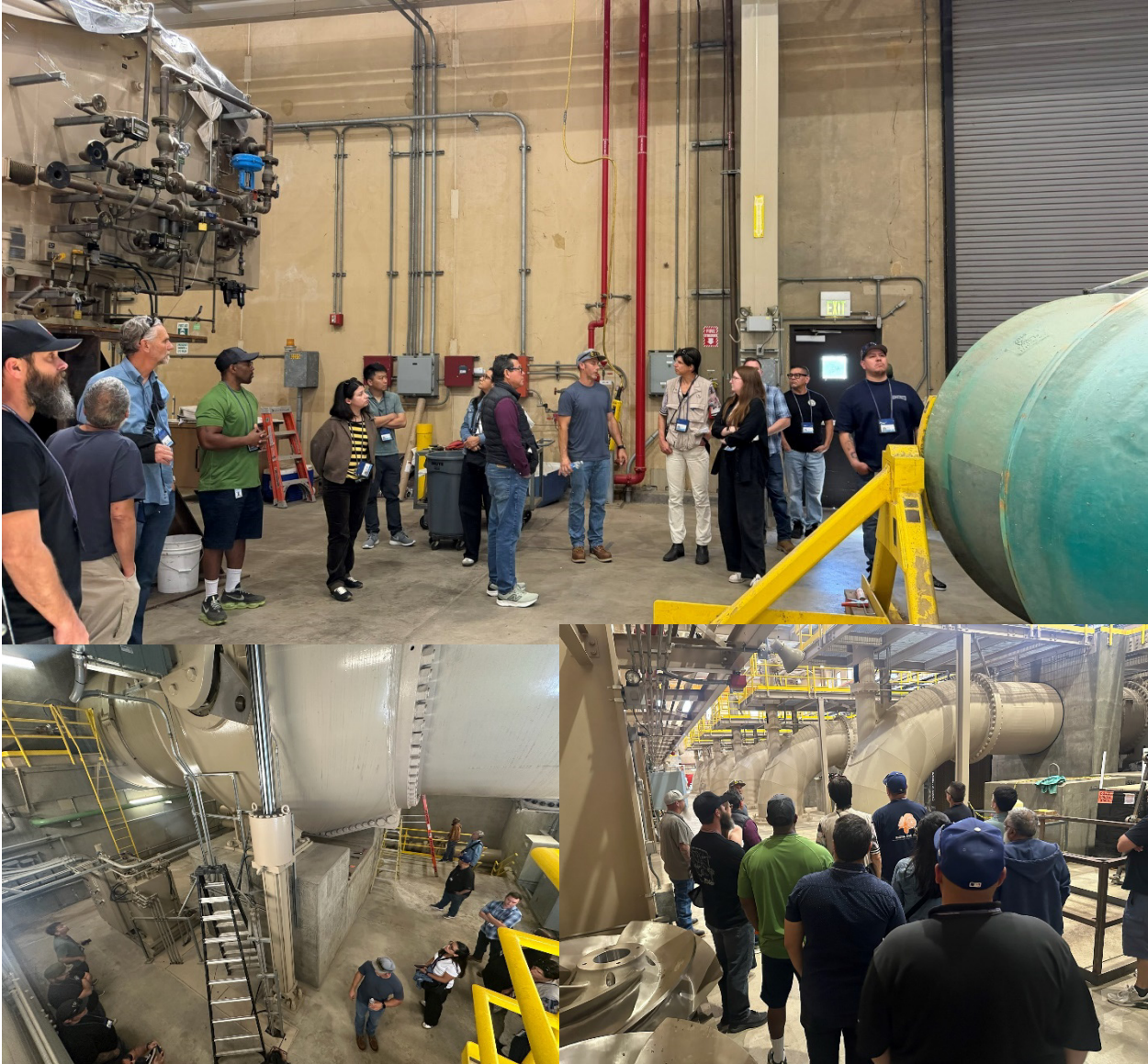
Photo by Brian Tubbs and Emily Liemsakul: Employees explore the inner workings of the Wadsworth Pumping Plant at Diamond Valley Lake.
