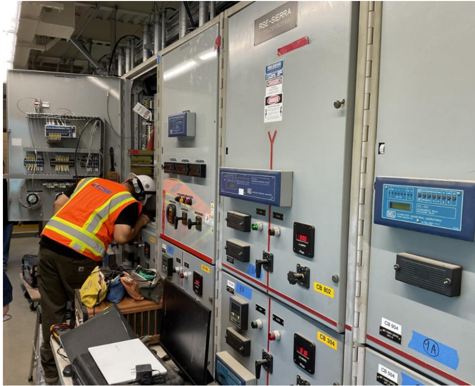
Mills Electrical Upgrades—ORP Switchgear New Door Testing
