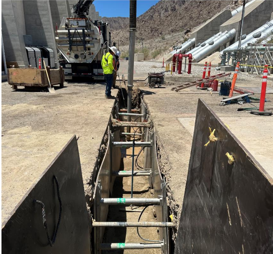
CRA Storage Buildings—Julian Hinds FMS 8 inch HDPE Fire Water Line Trench Hydro Excavation
