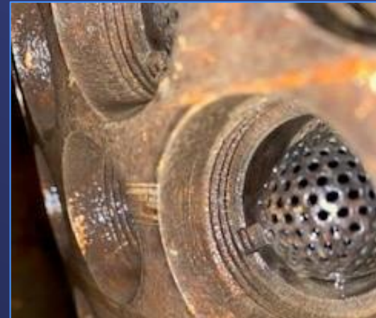
Jensen Plant Ozone Cooling System Strainer
