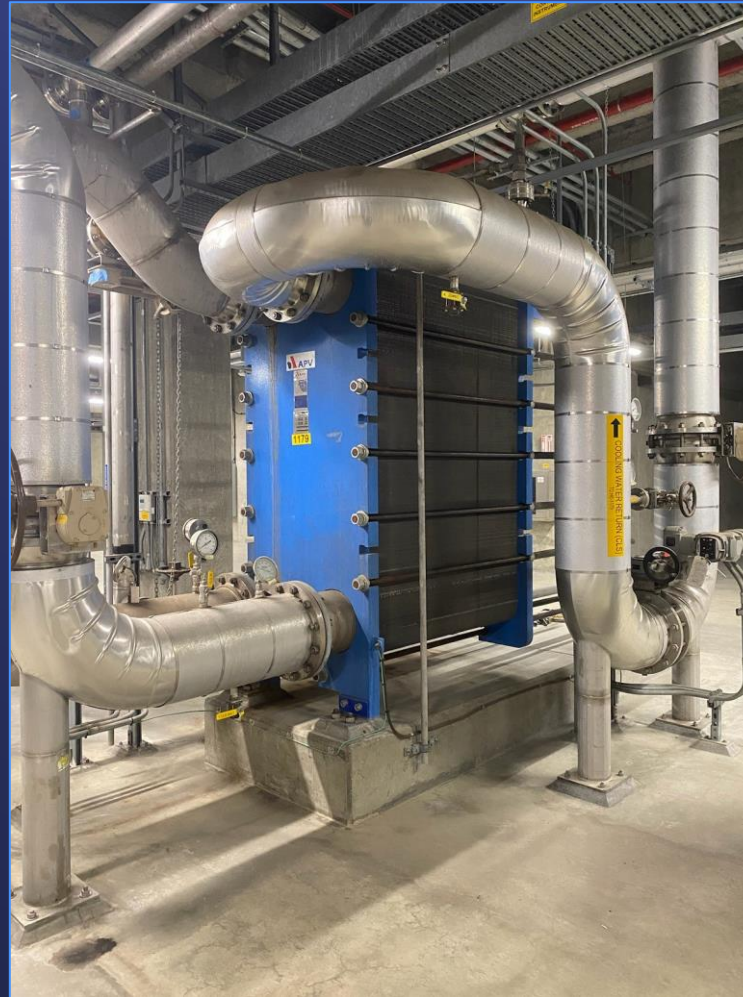
Ozone Cooling System Heat Exchanger
