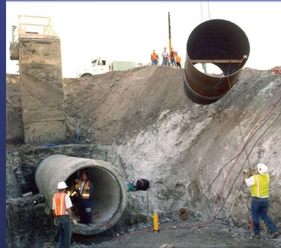
1999 Allen-McColloch Pipeline Break
