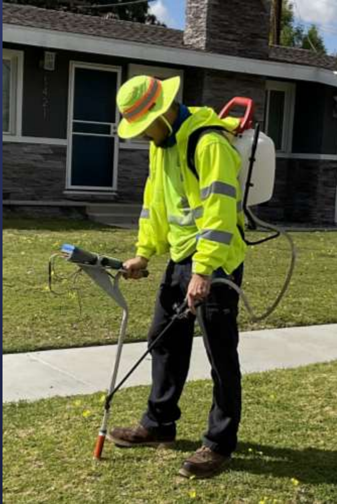
Stray Current Monitoring
