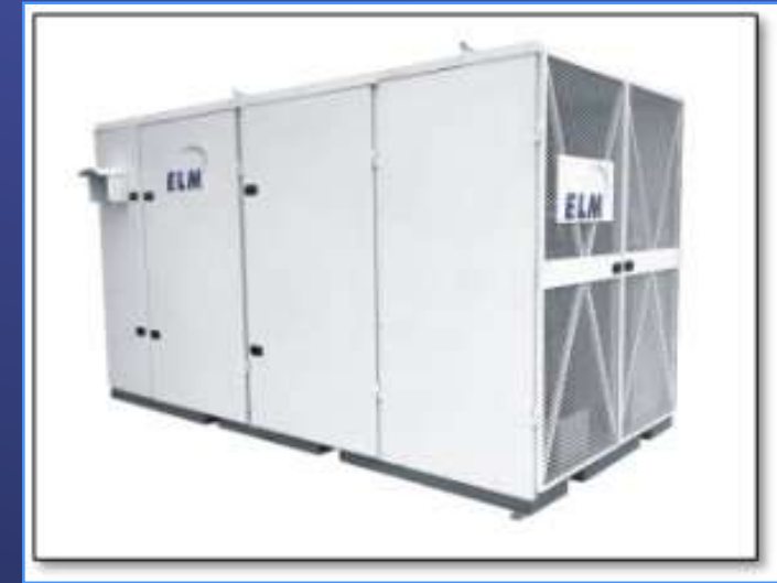
Typical Battery System
