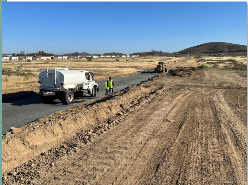
Contractor installing crushed aggregate base for fire access road at Skinner WTP
