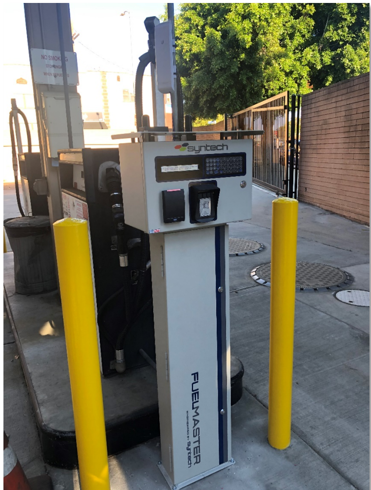
Pilot fuel management kiosk at Sunset Garage
