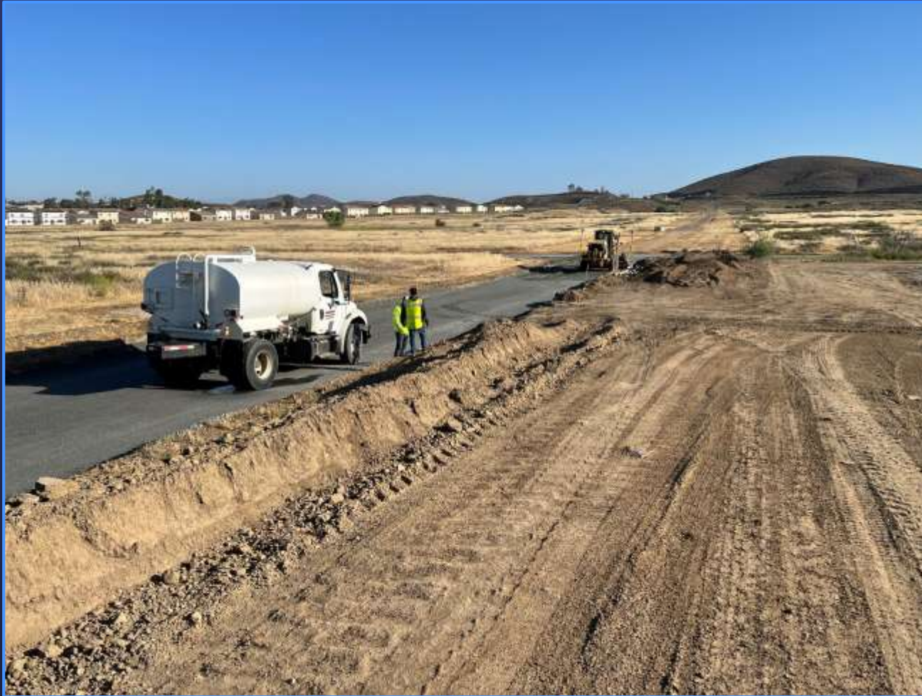
Contractor installing crushed aggregate base for fire access road at Skinner WTP
