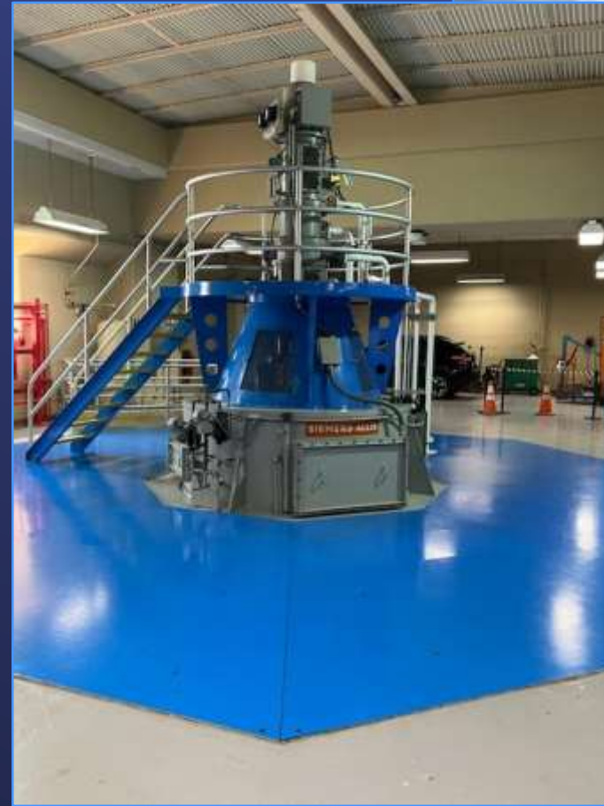
SWP Oso Pump Plant
