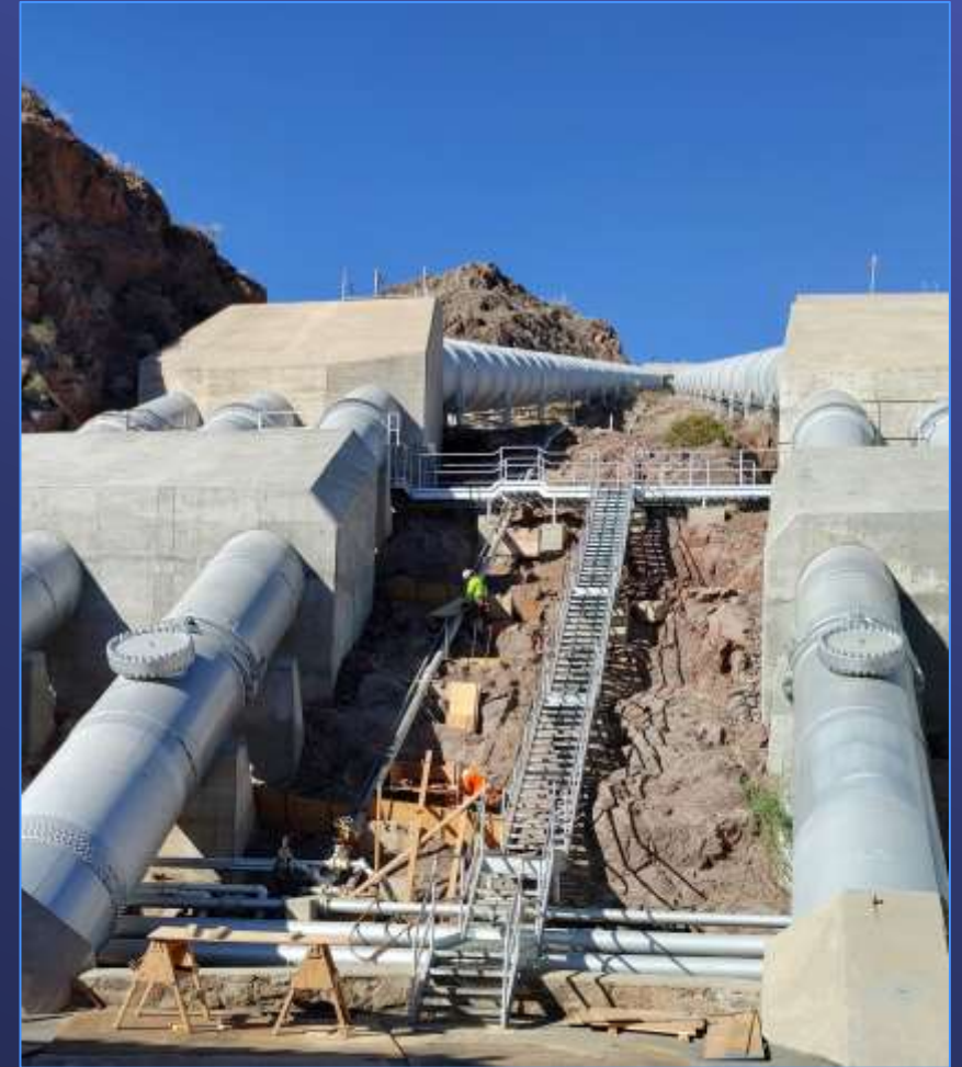
Contractor prepared subgrade to install above-ground conduit support pedestals at Intake Pumping Plant
