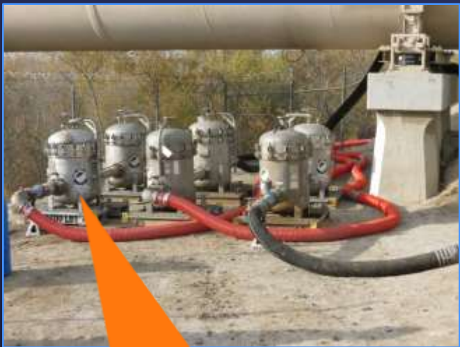
Quagga Filters for Dewatering
