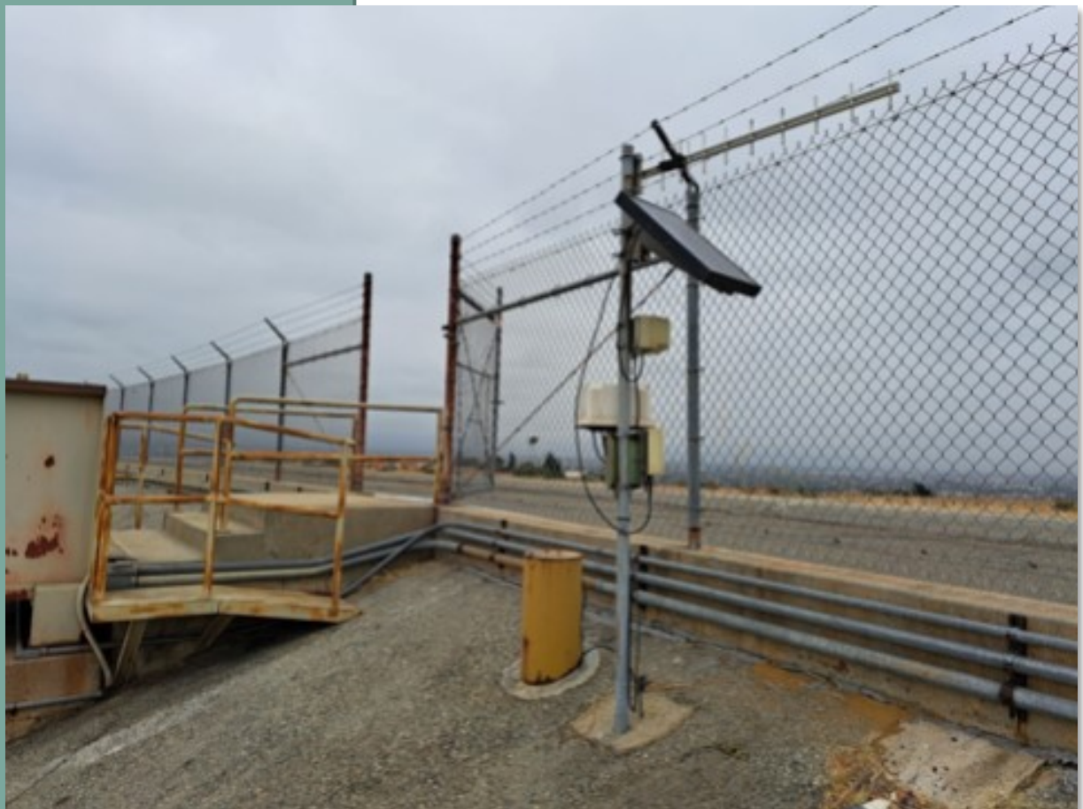
Existing dam monitoring station at Garvey Reservoir
