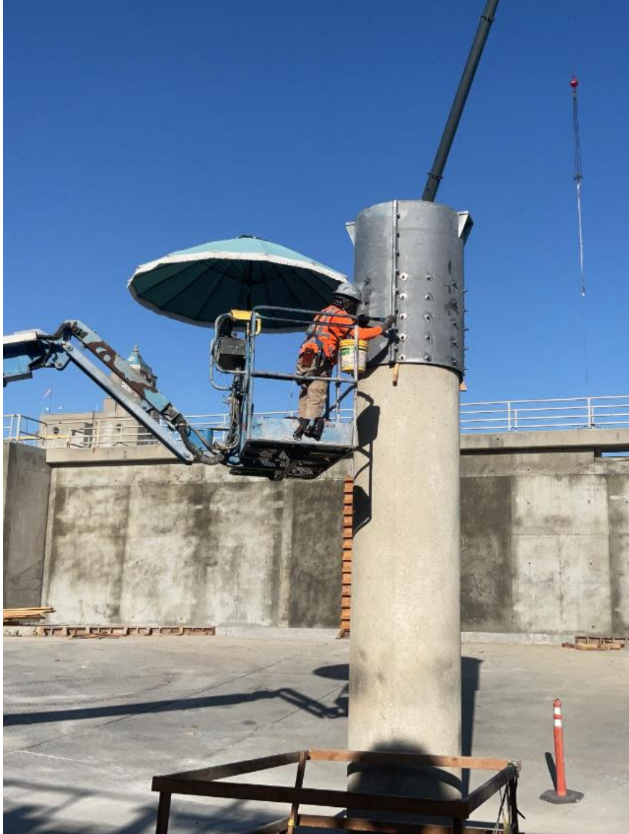
Weymouth Basins 5–8 and Filter Building No. 2 Rehabilitation – Installing the clarifier column cap at Basin 6, view to the west.
