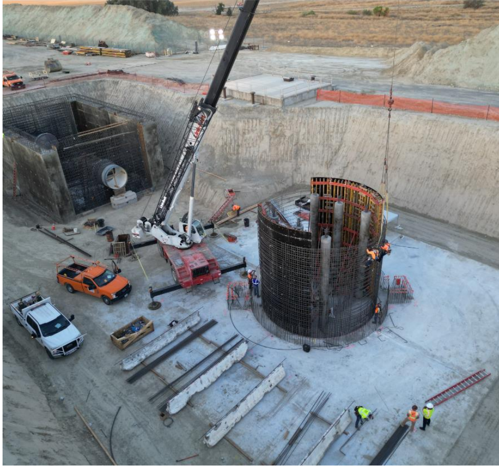
Inland Feeder - Badlands Tunnel Surge Protection – Installation of Rebar at the Surge Tank Foundation
