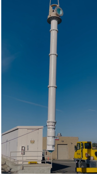
Staff installing a rebuilt surface wash pump at Mills plant
