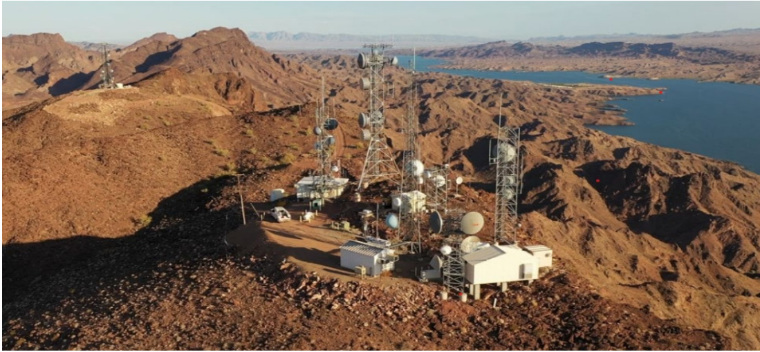
Black Metal Mountain Communications Site
