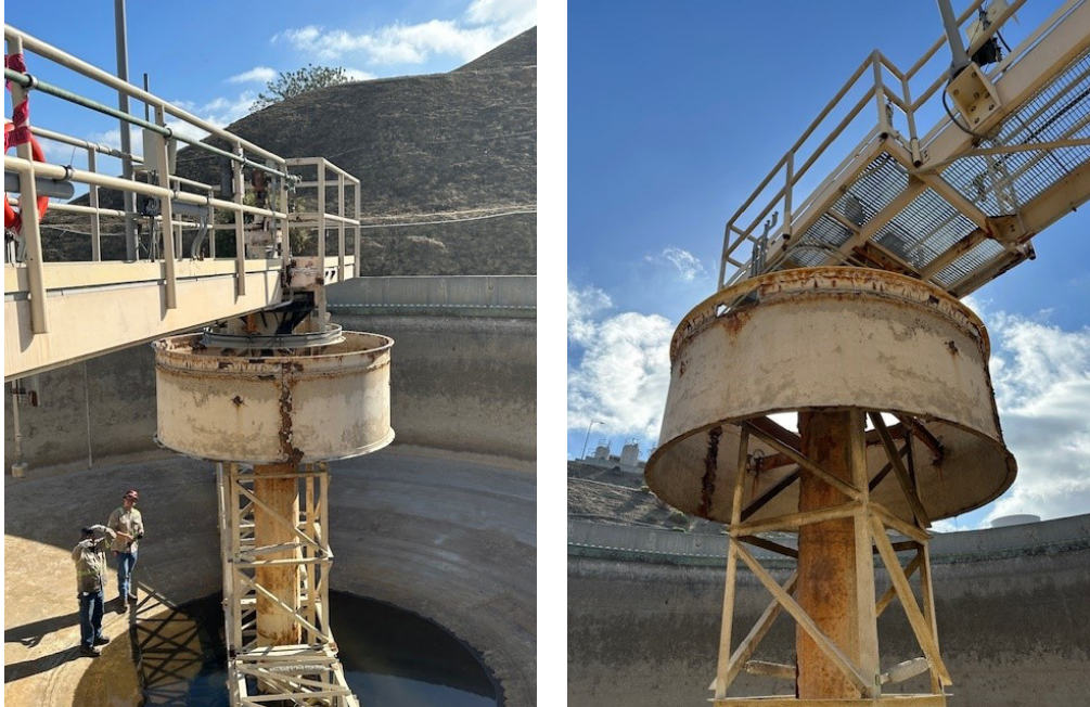
Staff inspecting the sludge thickeners at the Diemer plant
