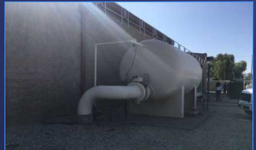
SBVMWD's Surge Mitigation System
