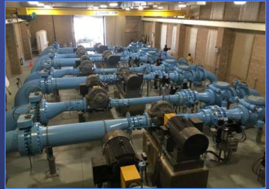
SBVMWD's Foothill Pump Station
