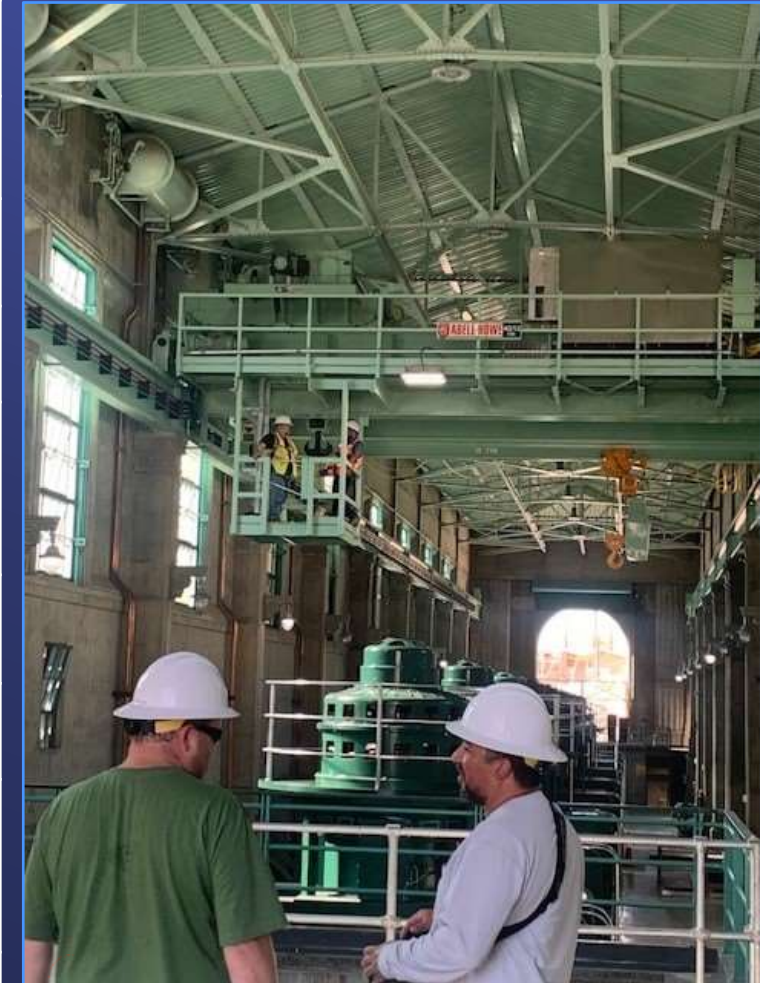
Iron Mtn. Pumping Plant
